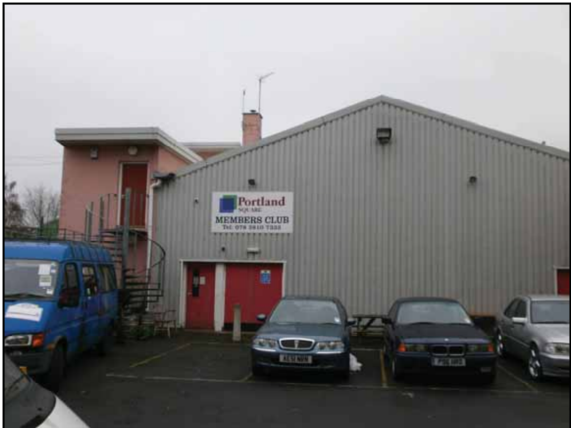
Pl. 4. The corrugated steel, gable ended, extension at the rear of the office building from the car park
