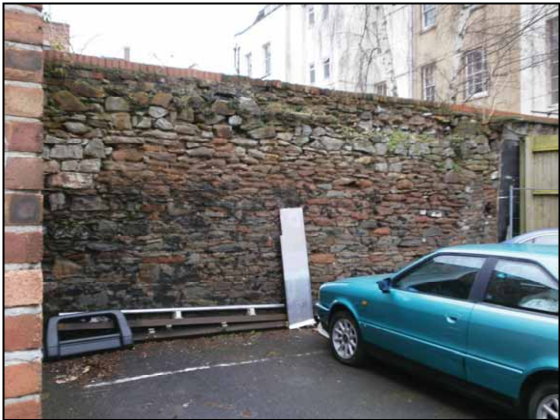
Pl. 20. The older stone and brick walling at the rear of the car park from the car park.
