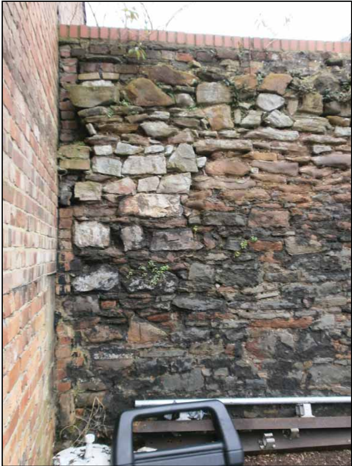
Pl. 21. Detail of the end of the wall as it abuts the gable end wall of the garages. This shows the irregular courses and use of different stone and brick types.
