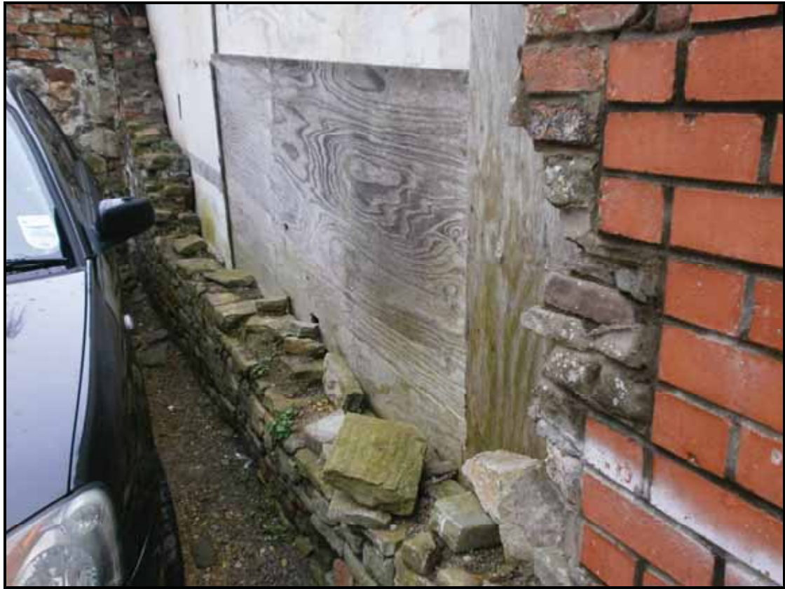
Pl. 9. The damaged walling on the south west side of the small garage
