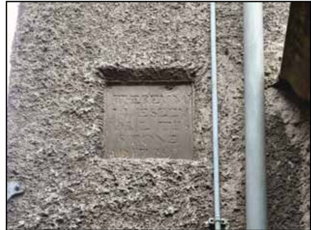
4. The inscribed foundation stone of the New Room, almost certainly no longer in its original position, but now placed high up at the NE corner of the northern wall. It seems to read: "The Rev M: J: Weseey [sic] MA [or AM] L[ai]d this stone 1739". Note the depth of the concrete render as revealed by the inseting of the stone into the underlying fabric of the wall.
