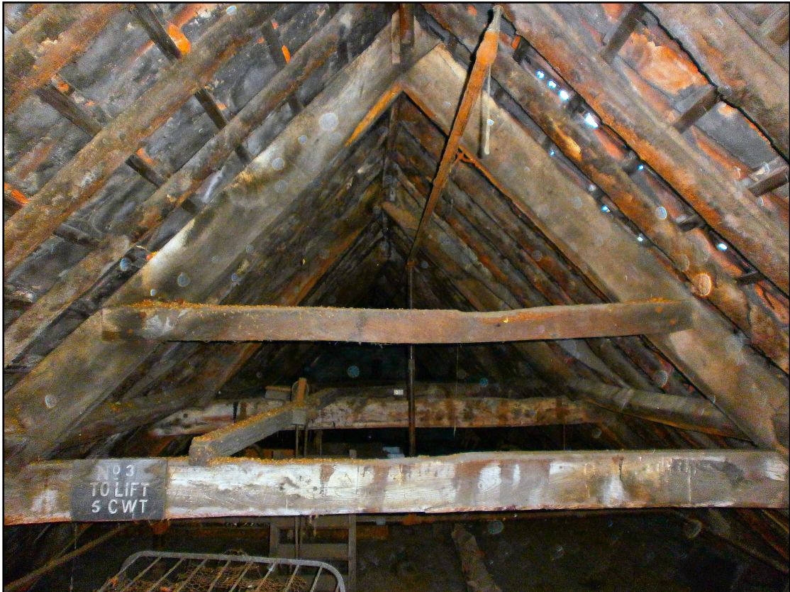
Frontispiece: part of the roof structure, which is probably original, within one of the surviving historic warehouse units of the Harris building.
