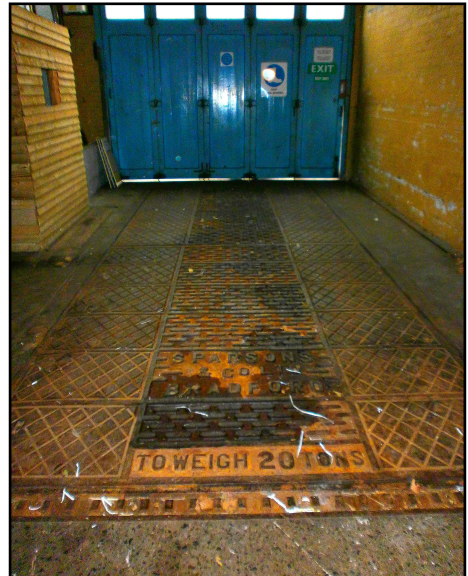
2. The weigh-bridge installed in the ground floor of the rebuilt warehouse units 1 and 2 after the fire of the mid 1950s. The large folding doors in the background open out onto Farr's Lane. View to north.
