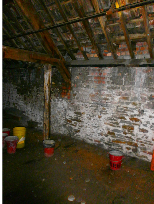
7. Indications of blocked up openings showing in upper internal wall fabric of Units 3 and 4.
