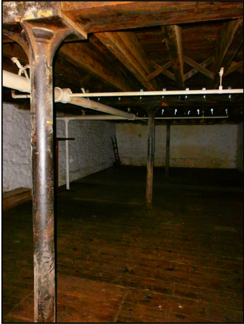
6. Iron columns and possibly original floor planking in upper storey of Units 3 and 4. View to S.
