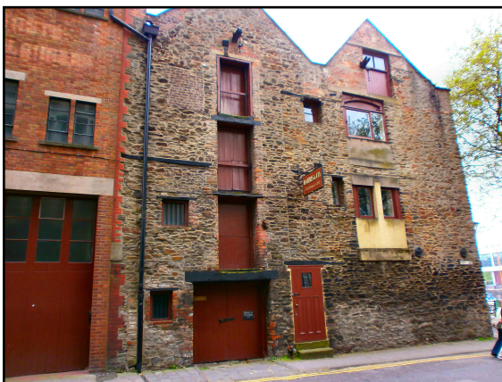
5. External northern elevation onto Farr's Lane of the historic elements units 3 and 4, showing at least one blocked opening, a defunct lintel, and other clear indications of structural sequence. View to SW.
