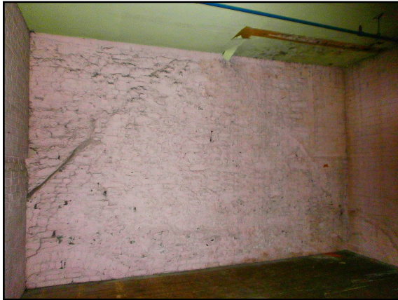
1. Impression of the roof line of the southern end-gable wall of one of the original units (1 and 2), preserved on the third storey within the rebuilt section of the warehouse following the fire of the mid 1950s. View to SW.
