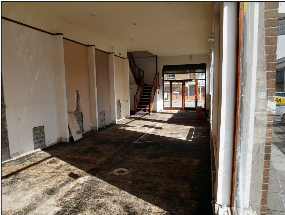
2. View from inside the ground floor 'reception' area of the building, with extensive glazing forming much of the frontage onto Redcliffe Street (to right of frame). In the background, to the left of the door, a set of wooden stairs leads up to office space at first floor level. View to NNW.
