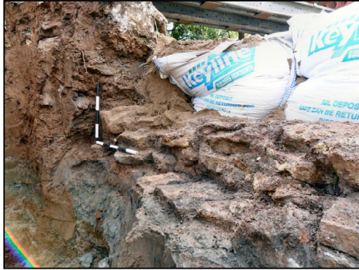
g) View of rear (north) elevation of Wall 518, showing Contexts 501, 500 and 503, from north-west. Scales: 500mm.
