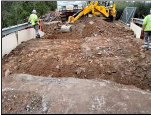
a) View of arch of Bridge, after removal of modern road surface, facing north, showing Context 520 to right of frame and Context 521 to left. No scale.
