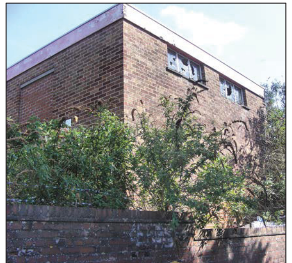
d) Building to rear (west) of site, with overgrown scrub in foreground, from north-west.
