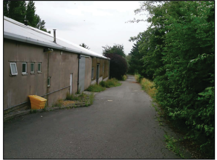
b) External view of west wall of warehouse at northern end of site, and adjacent road, from north. Note that the ground slopes down from a maximum height of approx. 125m aOD (in the foreground) to 120m aOD at Pipehouse Lane, to the south.
