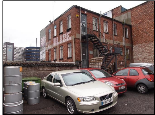
2) Exterior view of the rear of the three-storey brick building sited in the extreme southwest of the study area and butting No. 53, looking south
