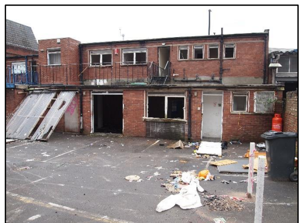
6) Rear view of the two-storey brick and concrete structure with railed roof area and loading bay door to grocer's shop, looking southeast
