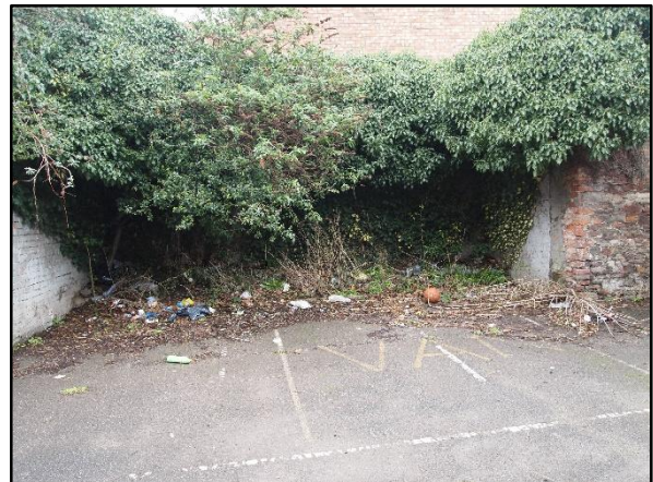
12) View of the heavily overgrown recess in the northwest boundary wall of No. 83 where earlier masonry is preserved, looking northwest
