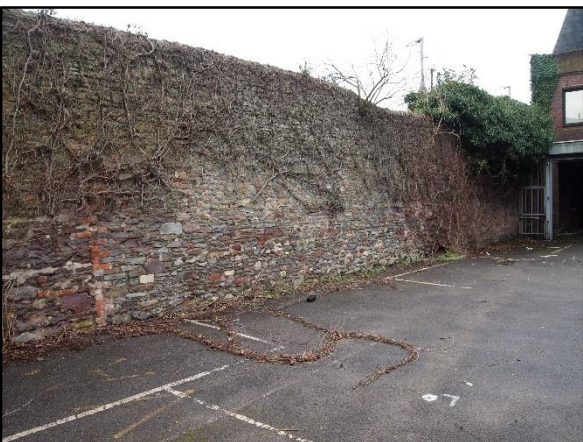
11) View of the multi-phase masonry wall on the northeast boundary of the yard at the rear of the police station (No. 83), looking east
