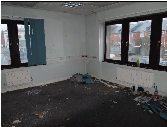
9) Interior view of a typical room in the former police station (No. 83) with some squatters' debris, looking west
