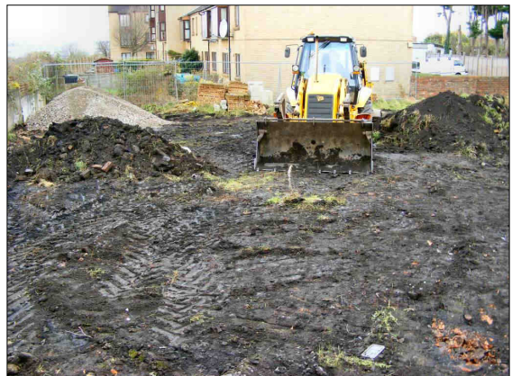
f. View of the Study Area after completion of the remedial ground works, looking west.
