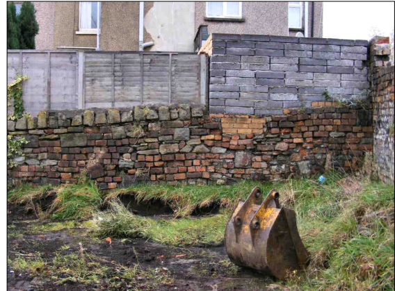
d. Reused bricks in the northern boundary wall of the southeast corner Study Area, looking north.
