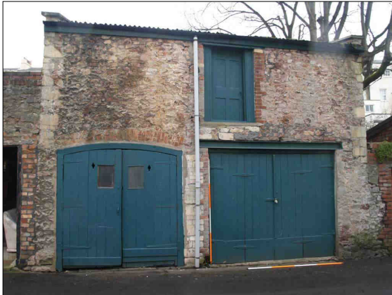
a. The southern face of the Coach House fronting Vyvyan Road, looking north. Scales 2 m by 2 m.
