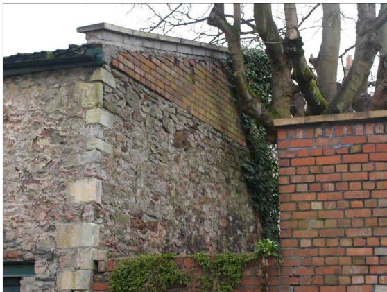
c. Detail of the east face of the Coach House, looking northwest. No scale.
