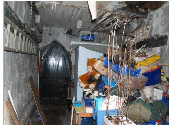
d. Ground floor interior view showing ceiling and former balcony supports over garden door, looking north. Scale 2 m.
