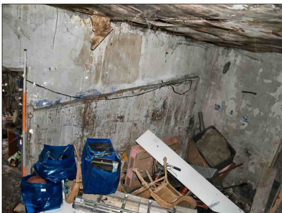
e. View of the former stables area, showing stalls and water damaged ceiling boards, looking northwest. Scale 2 m.
