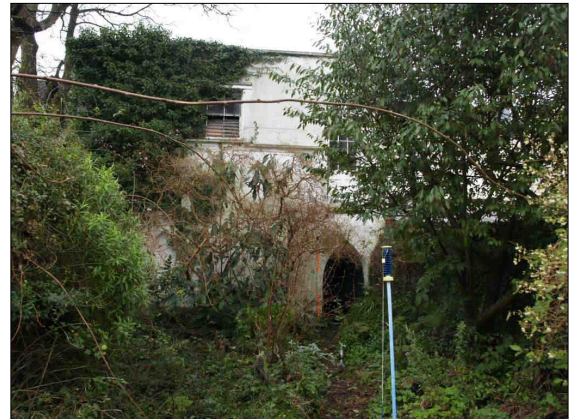
b. The northern face of the Coach House, looking south from the garden of No. 16. Scale 2 m.
