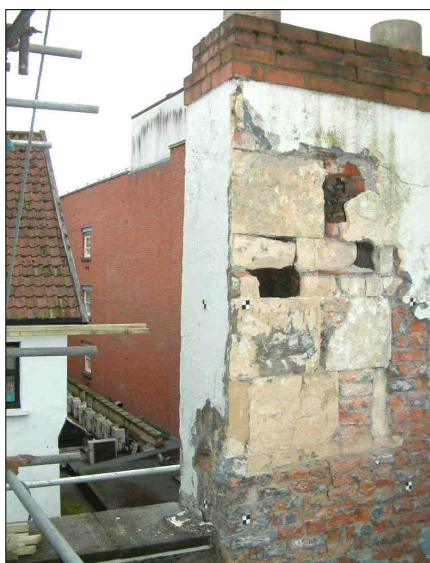
e. North and west faces of the chimney, looking southeast. Targets on north face 1 m apart.
