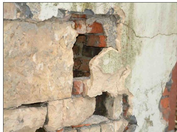
f. Detail from the interior of the earlier flue, seen through a void on the west face, looking southeast. No scale.
