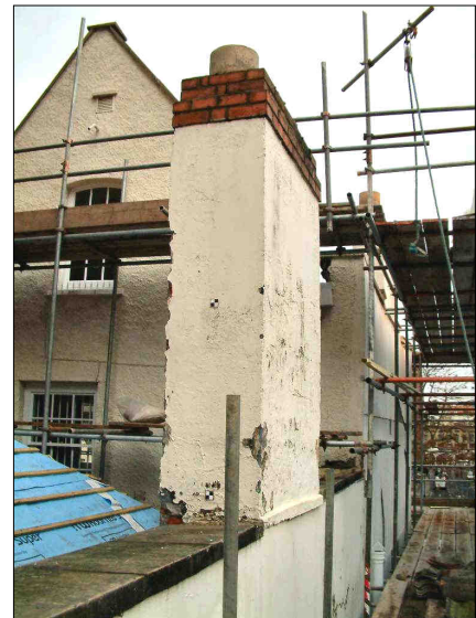
b. The south and east faces of the chimney, looking northwest. Targets 1 m apart.
