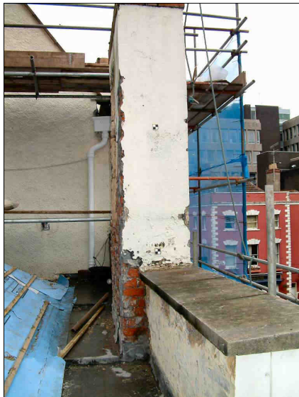
c. The south face of the chimney, looking north. Targets 1 m apart.
