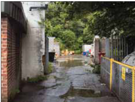
Plate 3: electricity substation adjoining the garages and workshops to east of the engineering works, viewed from the southwest
