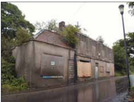
Plate 5: Crews Hole Road frontage of the now derelict former 19 th century public house, the Lamb Inn, viewed from the southwest
