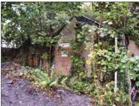
Plate 7: detail of the overgrown eastern part of the derelict former inn, viewed from the south
