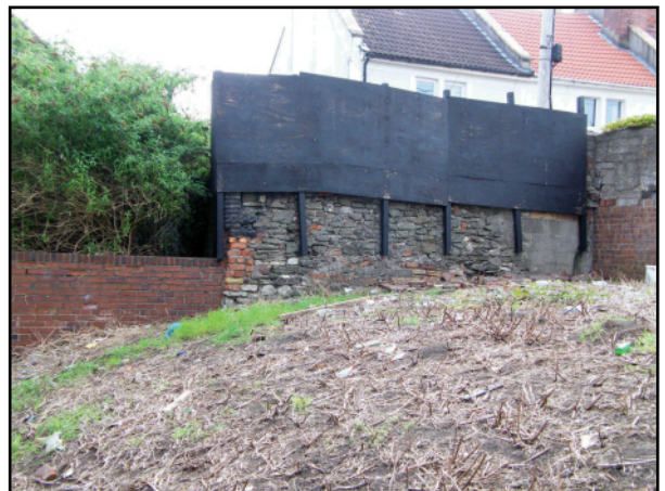
16. Surviving stone wall representing original south-west boundary of No. 20 Victoria Place, now removed. Extreme south-east corner of development site, view to north-east.
