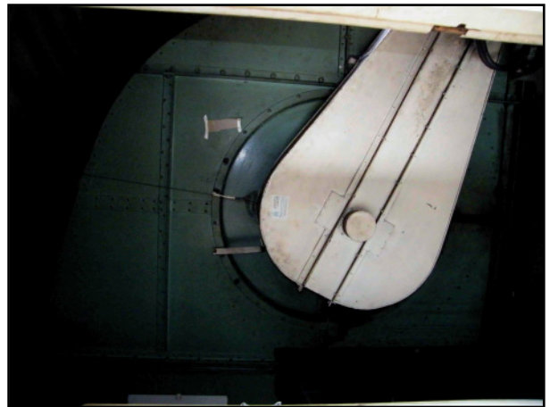
15. Gala Bingo Hall, detail of original and in situ (1941?) air extraction machinery.
