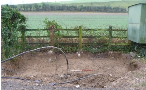
Plate 3. Generator compound (from NE; 1m scale)
