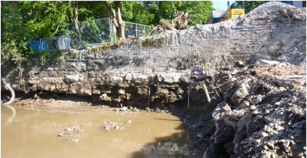
Plate 5. North facing elevation of south sluice wall showing timbers (103) surrounded by weir stonework (104) with more recent wall above (2 x 1m scales; from N)
