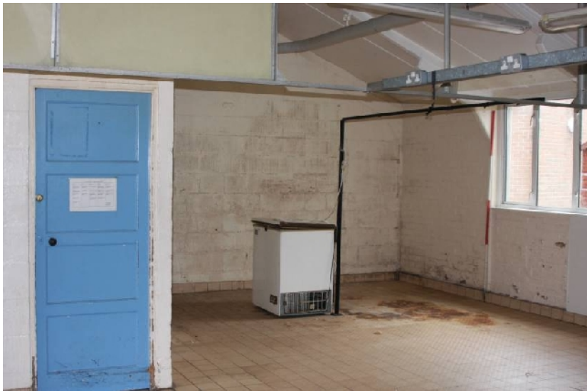
Plate 46. Kitchen Area within MOWP Hut (D) detailing floor (scale 2m, from NE)
