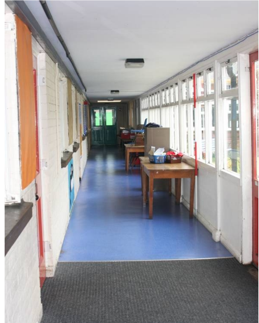
Plate 17. The 'Cloister' enclosed by later wall and windows (scale 2m, from E)
