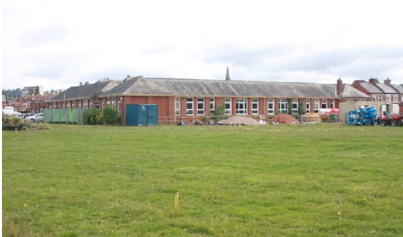
Plate 1. West and south ranges of main school building showing roof structure (from SW)
