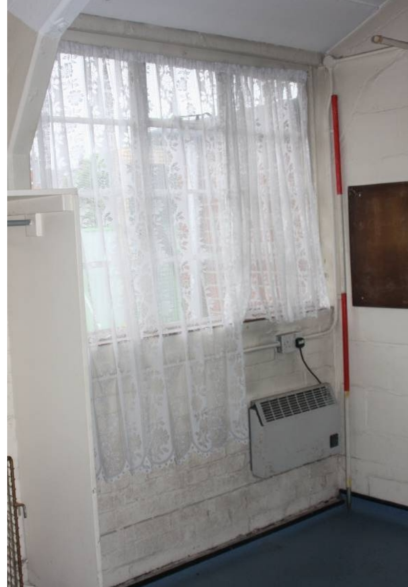
Plate 47. Detail of metal windows within MOWP Hut (D) (scale 2m; from NW)
