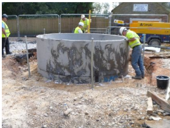
Plate 3. Sewage pumping station (from NE)
