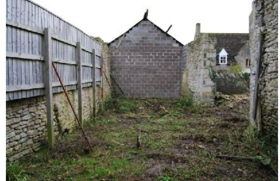
Plate 2. B1 interior showing conversion of east end outside of the Site (from W)
