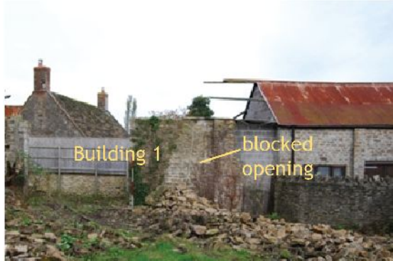
Plate 1. B1 exterior south elevation showing partial conversion of the eastern end (from S)
