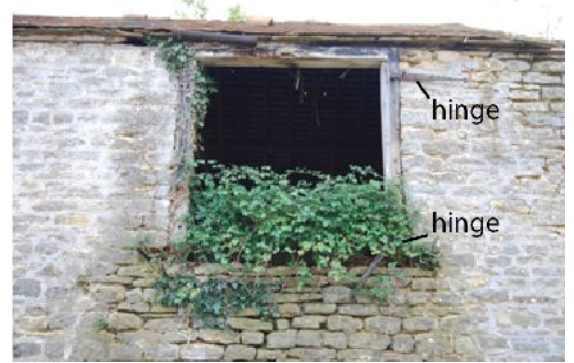
Plate 26. B5 exterior north elevation, blocked opening & window above with hinges (from N)
