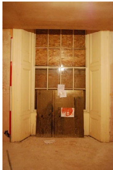
Plate 9. Exemplar window with wood panelling in building A (from W; 2m scale)
