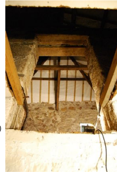
East side of roof in building I observed through hatch in ground floor ceiling (from W)
