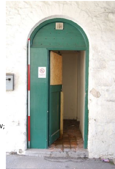
Doorway from coaching entrance E into building F (from S; 2m scale)
