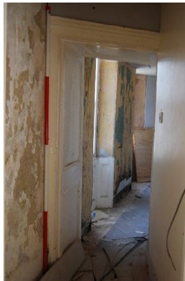
Corridor in first floor of building F showing curve in building (2m scale; from NW)
