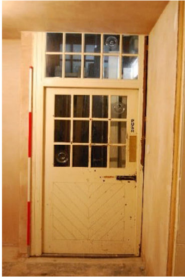
Internal door off hallway from main entrance in west elevation of building A (from S; 2m scale)
