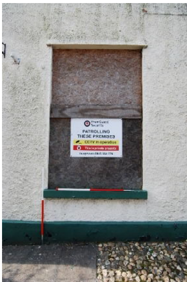
Window in position of old doorway at S end of east elevation of building A (from E; 2m scale)
