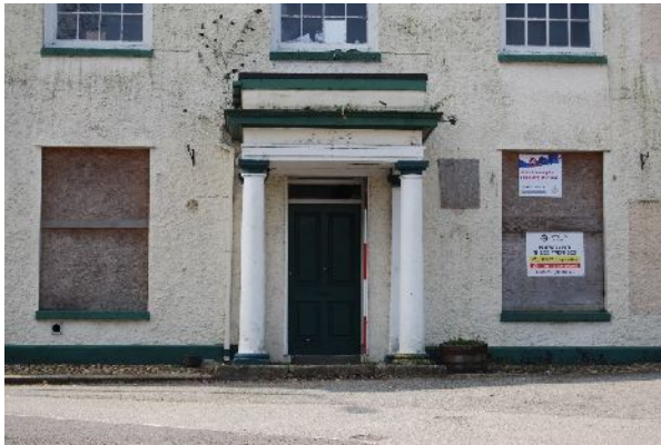
Main entrance in east elevation of building A (from E; 2m scale)
