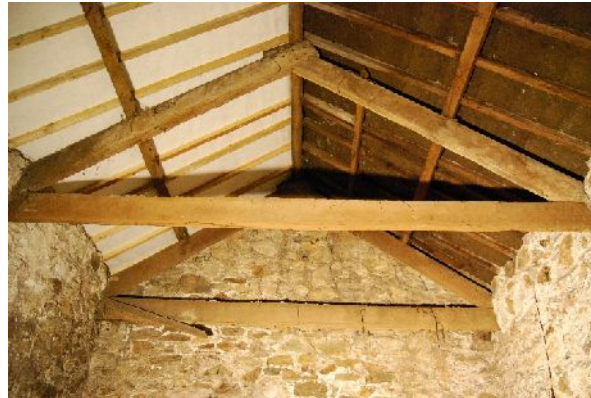
West side of roof in building I observed through hatch in ground floor ceiling (from E)
