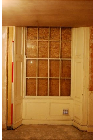
Exemplar window with wood panel surround in west elevation of building A (from W; 2m scale)
