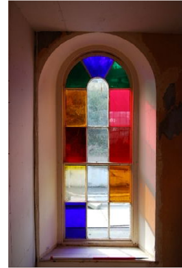
Interior of round-headed window in east elevation of building A (from E)
