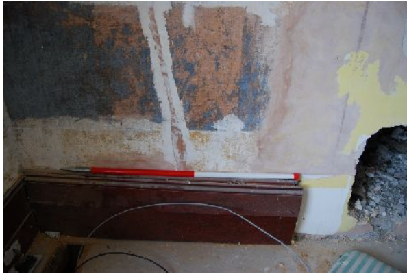
Traces of earlier décor in first floor bedrooms of building F (1m scale)
