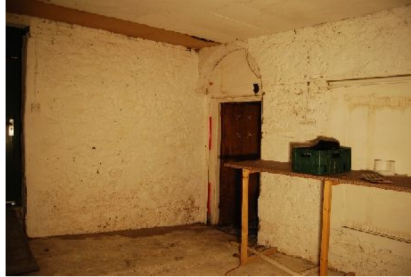
Ground floor of building I with round-headed door (from SE; 2m scale)
