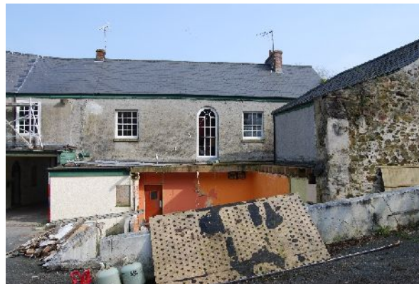
West elevation of building A following removal of modern extension (from W; 2m scale)
