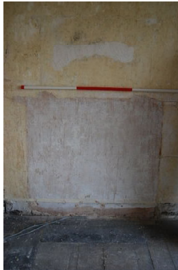
Blocked fireplace in first floor bedroom of building F (1m scale)
