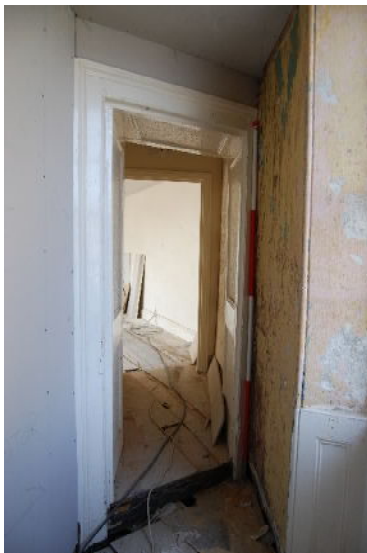
Corridor in first floor of building F showing curve in building (2m scale; from ESE)
