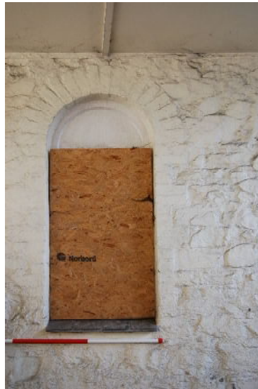
Blocked window on north side of coaching entrance E (within passage) (from S; 1m scale)
