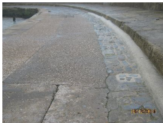
Plate 8. Re-instatement in Area 4 after duct trench works (from the NNW; photo by David Wilson)
