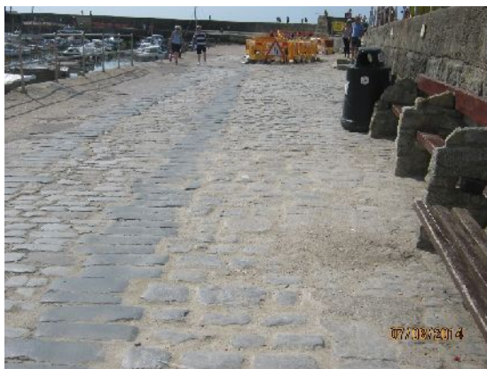
Plate 5. Re-instatement after duct trench works (from the N; photo by David Wilson)
