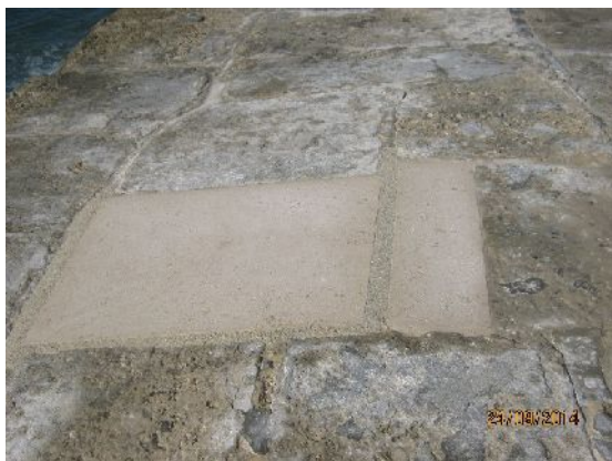
Plate 13. Replacement Portland Roach stone in Area 11 (from the N; photo by David Wilson)
