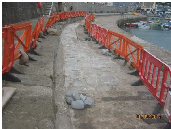
Plate 7. Re-instatement in Area 4 after duct trench works (from the SSE; photo by David Wilson)
