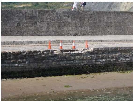
Plate 28. Damage to inner harbour wall in Area 5 (from E)
