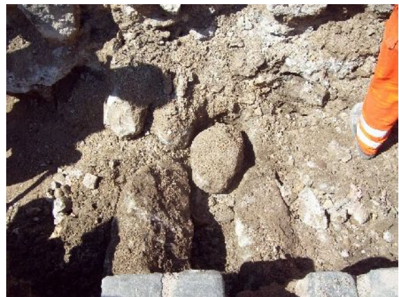
Plate 23. Earlier surface of large random boulders in duct trench, between 23m & 26.50m (from SW)
