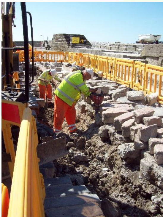
Plate 1. Open cut trenching in central area of main duct trench (from NNE)
