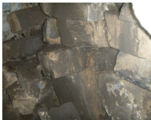
Plate 4. View inside collapsed culvert
