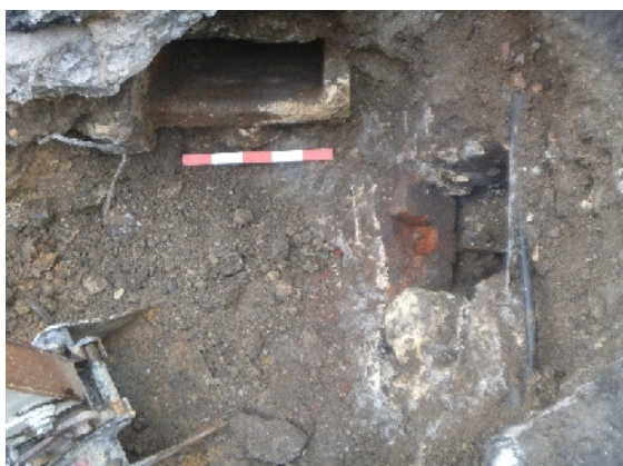
Plate 3. Iron grate & void in culvert (0.5 scales)
