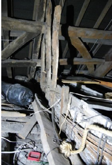
Plate 13. Purlins, arched wind-braces, lathe and plaster division with timber uprights (from SSW)
