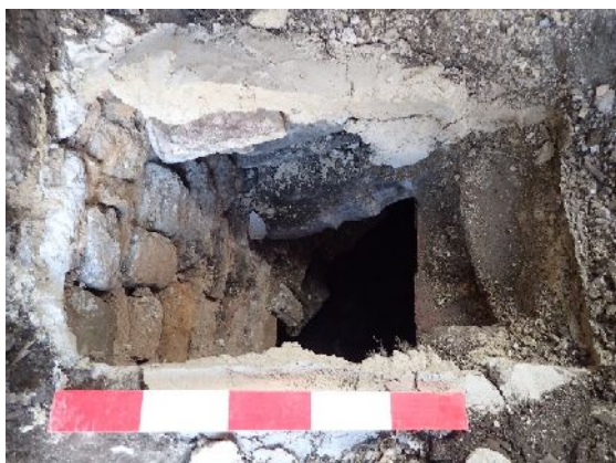
Plate 43. Brick retaining wall running north from NW corner of Institute (from N; 0.5m scale)
