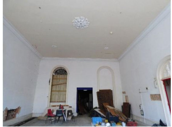
Plate 6. Ground floor Reading Room showing later doorway & blocked window (from S)
