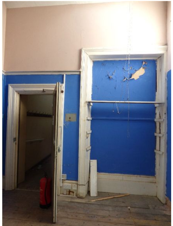
Plate 8. North Building before works showing blocked door & door to east corridor (from N)
