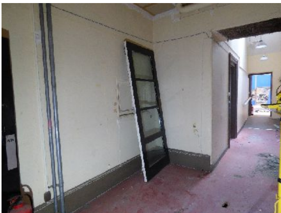
Plate 9. Lobby showing serving hatch to Reading Room & doorway to corridor (from S)
