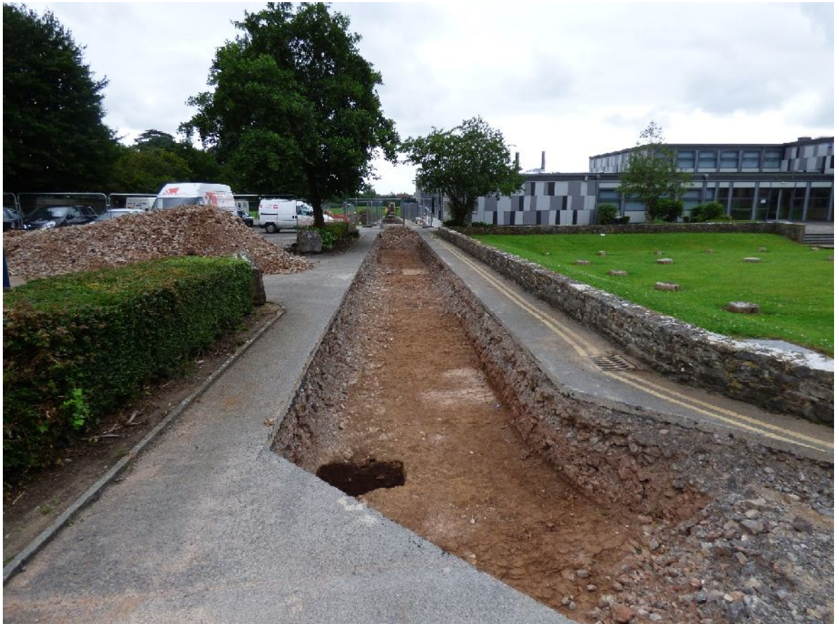
Plate 2. Tr1 with location of timber-framed East Hall on the right (from N)
