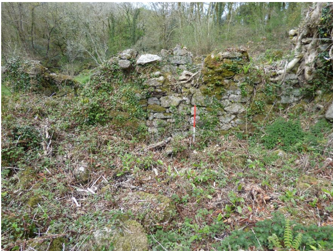
Plate 17. Southern cottage showing interior NW elevation with blocked doorway to Building B (from SE; 1m scales)
