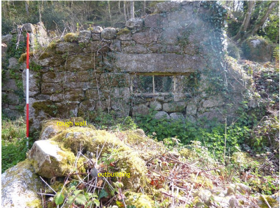
Plate 11. Building B - window in exterior SW elevation with wall & outbuilding to S (from NE; 1m scales)
