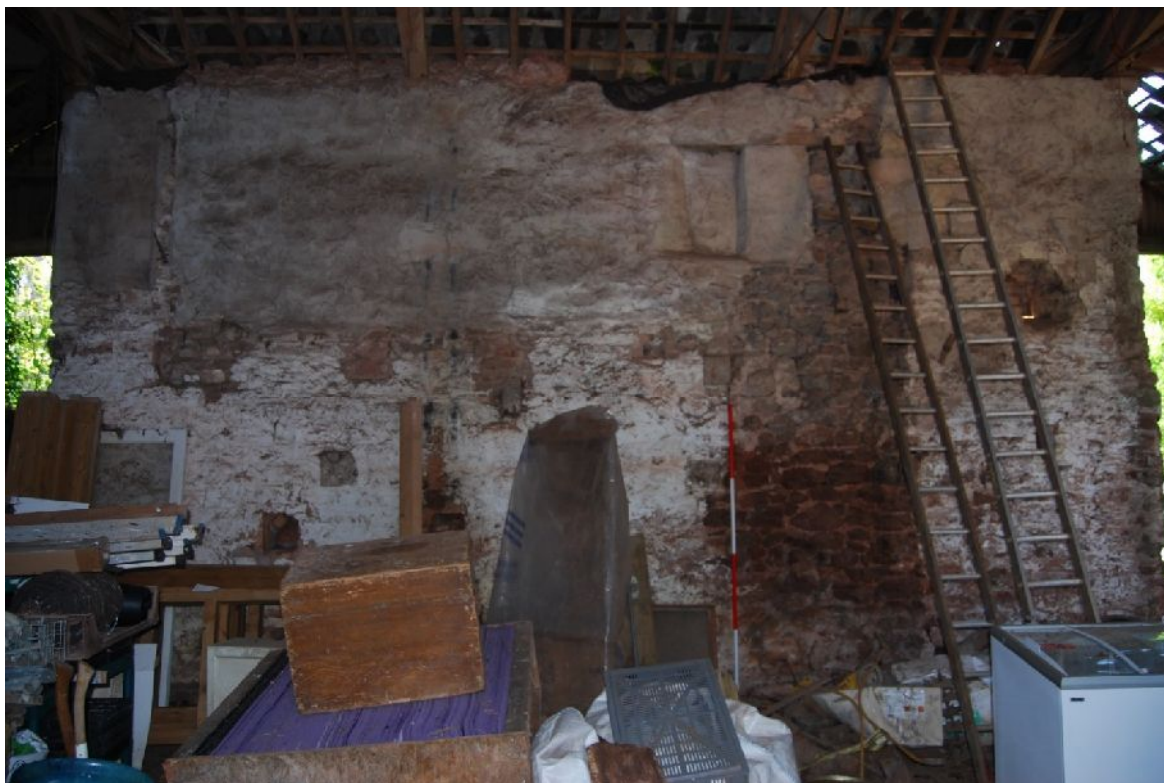
Plate 13. Central part of south-west interior elevation of B1 showing blocked window (from NE; 2m scales)
