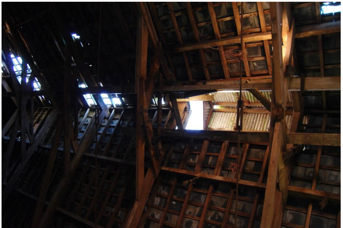
Plate 21. Roof of B1 showing scissor beam trusses & later corrugated iron ventilation structure on ridge (from below)
