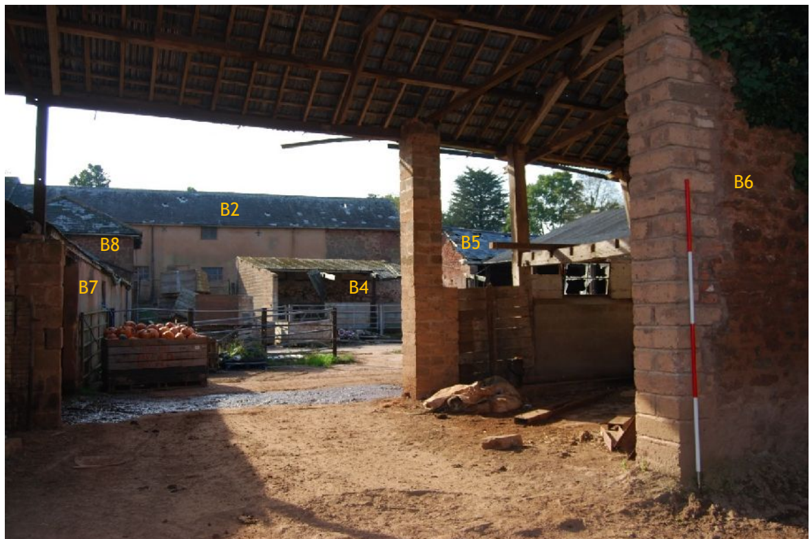
Plate 54. View from outside east range across farmyard to main barns (B1 & B2) (from ENE; 2m scales)
