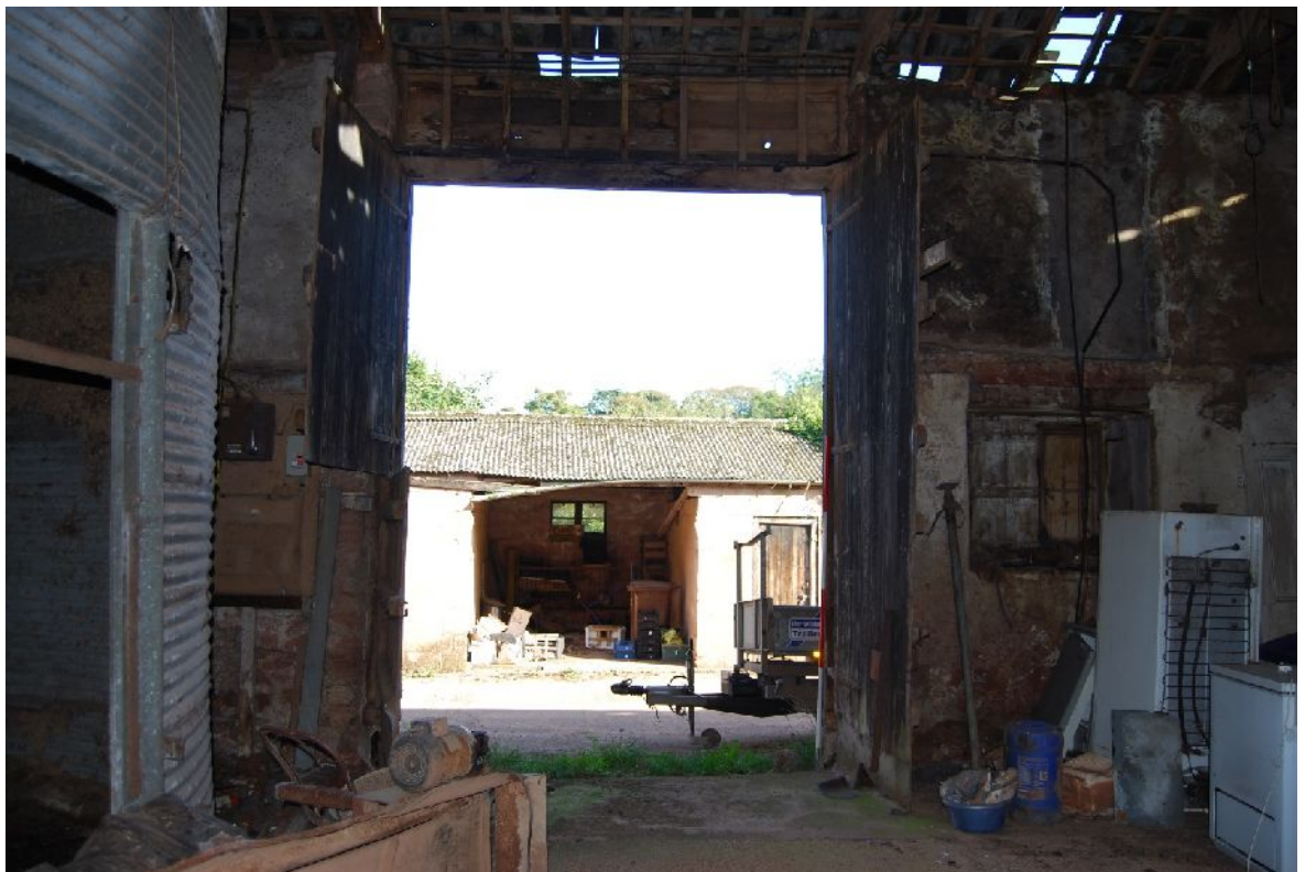
Plate 18. North-east interior elevation of B1 showing north full height door (from SW; 2m scales)
