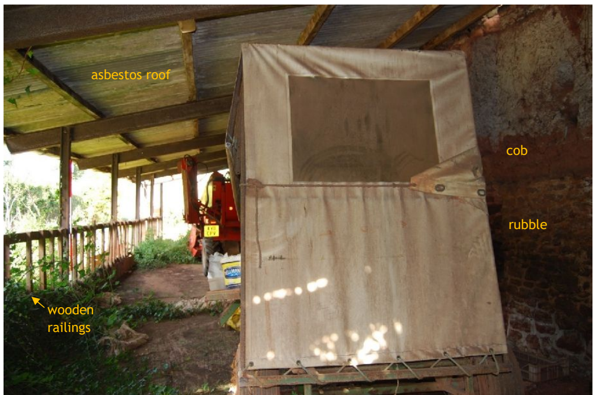
Plate 26. South-west side of B2 showing lean-to cattle shelter (from SE; 2m scales)
