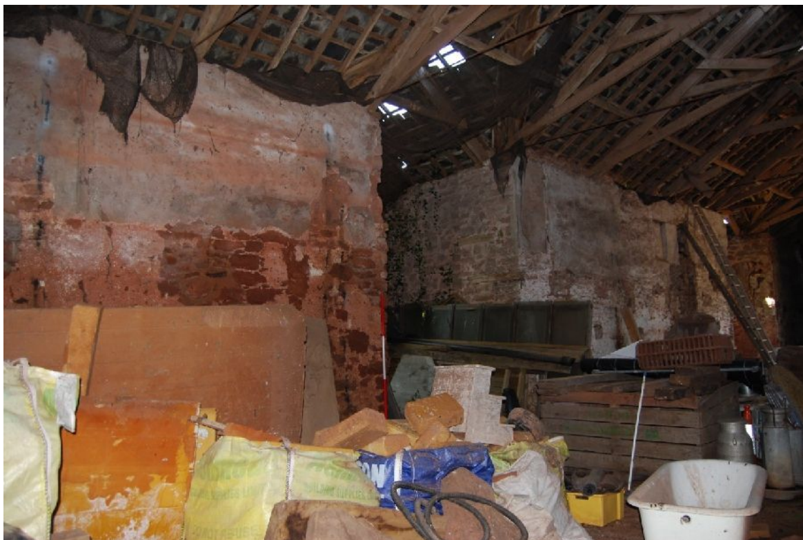
Plate 11. South-west interior elevation of B1 showing south porch (from ESE; 2m scales)
