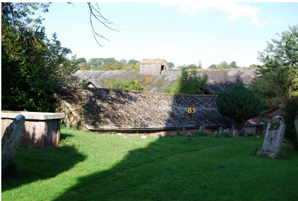
Plate 55. Roof of B3 adjacent to graveyard & roof of B1 beyond (from SSW)
