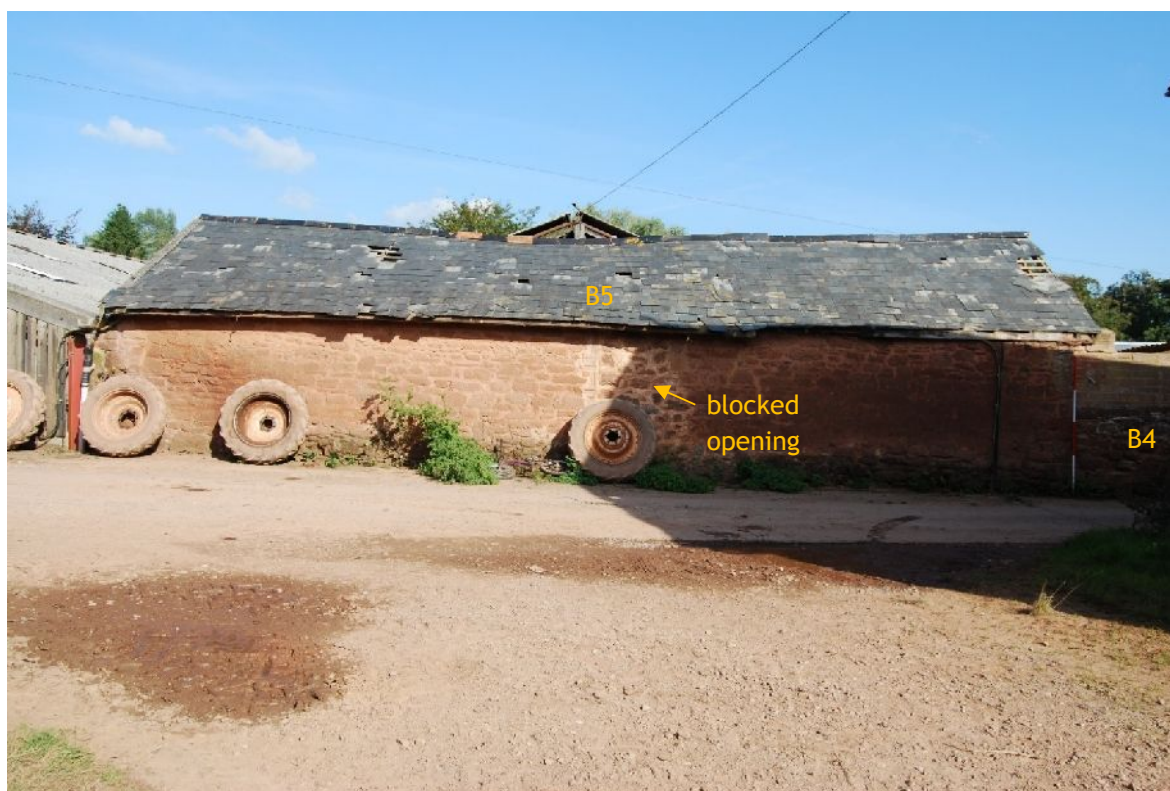
Plate 37. South-west exterior elevation of B5, continuing into B4 (from SW; 2m scales)
