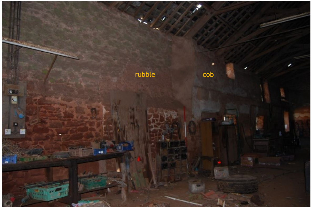
Plate 33. North-east interior elevation of B2 showing change in build at N end (from NW; 2m scales)
