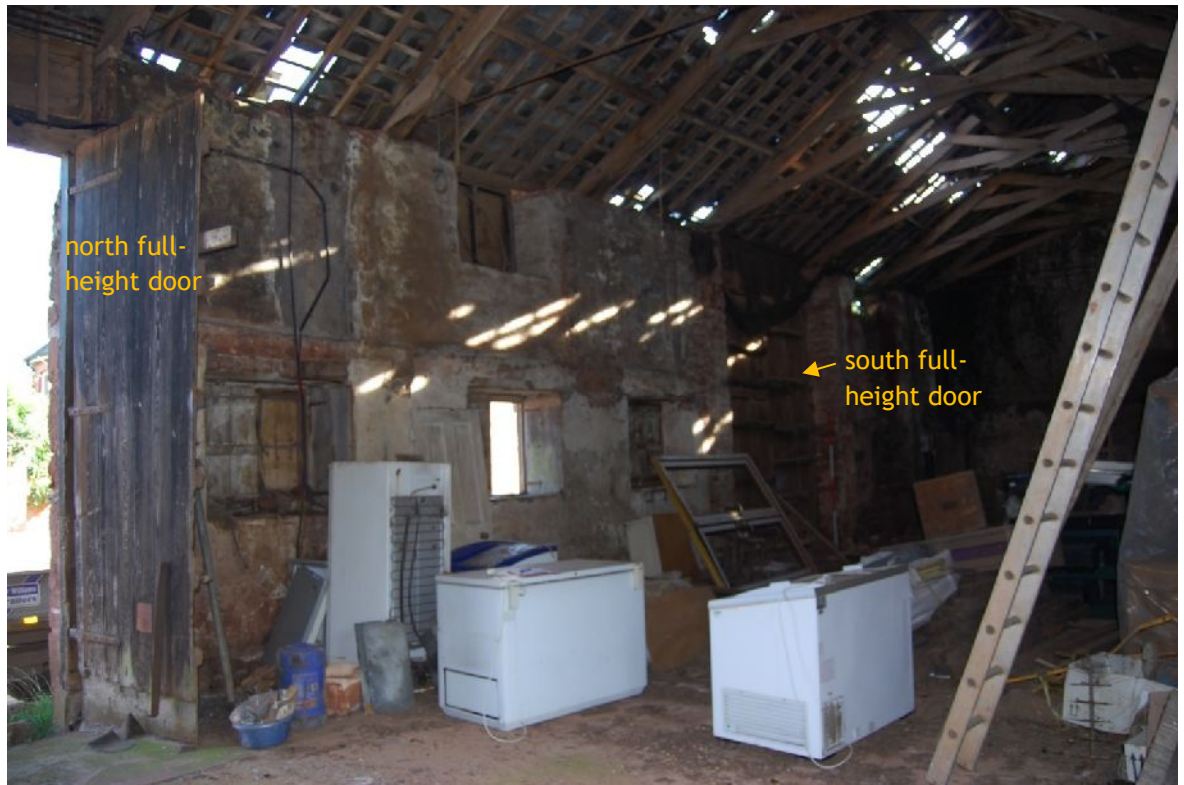
Plate 9. North-east interior elevation of B1 showing 4 shuttered windows (from NW; 2m scales)
