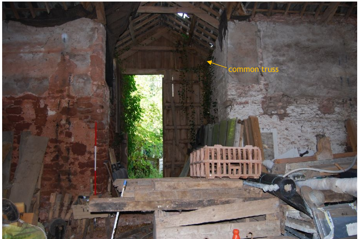
Plate 15. South-west interior elevation of B1 showing south porch with common trusses (from NE; 2m scales)
