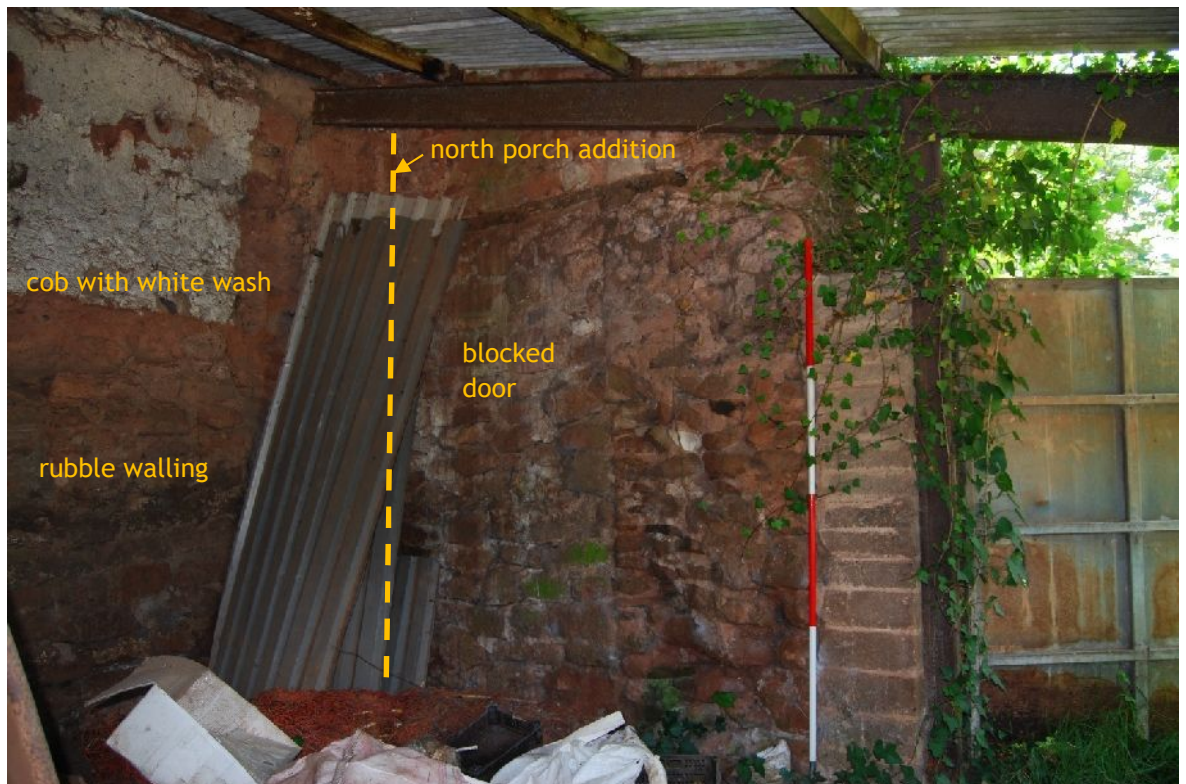
Plate 6. North-west side of added north porch of B1 against SW elevation (from NW; 2m scales)
