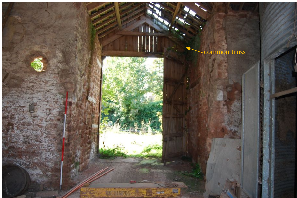
Plate 16. South-west interior elevation of B1 showing north porch with common trusses (from NE; 2m scales)
