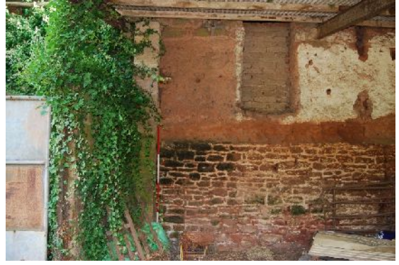
DSC 0024. South-west elevation of B2 at junction between modern blockwork & old fabric (from SW; 2m scales)
