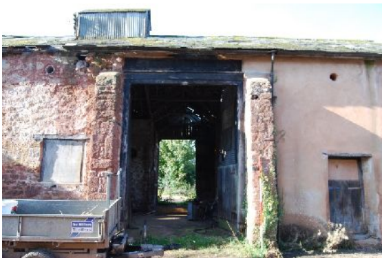
DSC 007. North-east elevation of B1 showing northern-most full height door (from NE; 2m scales)
