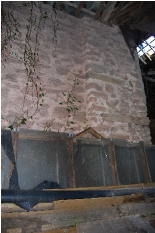
DSC 0055. North-west side of southern-most porch of B1, added to SW elevation (from WNW; 2m scales)
