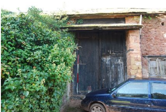
DSC 005. North-east elevation of B1 showing southern-most full-height door (from NE; 2m scales)
