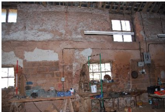
DSC 0075. North-east interior elevation of B2, near centre (from SW; 2m scales)
