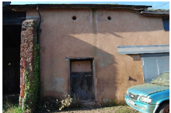
DSC 008. North-east elevation of B1 where it adjoins B2 (from NE; 2m scales)
