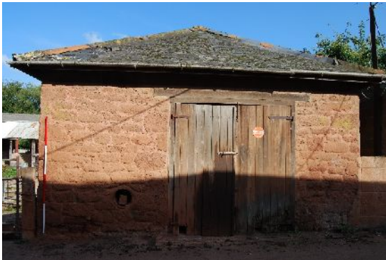
DSC 0088. South-west elevation of B8 bordering farm lane (from SW; 2m scales)
