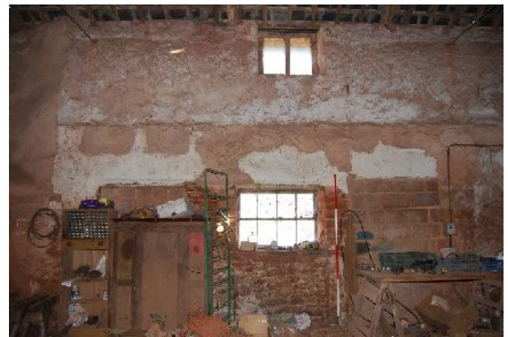
DSC 0074. North-east interior elevation of B2, along centre (from SW; 2m scales)
