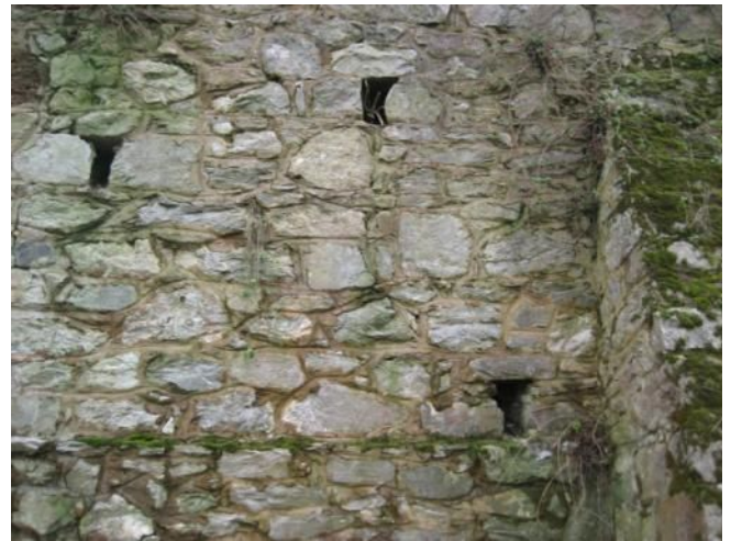
Plate 25. Voids in upstream elevation (looking SE)
