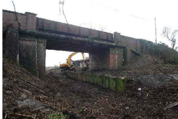
North elevation – focussed on west side with platform under bridge (from N)
