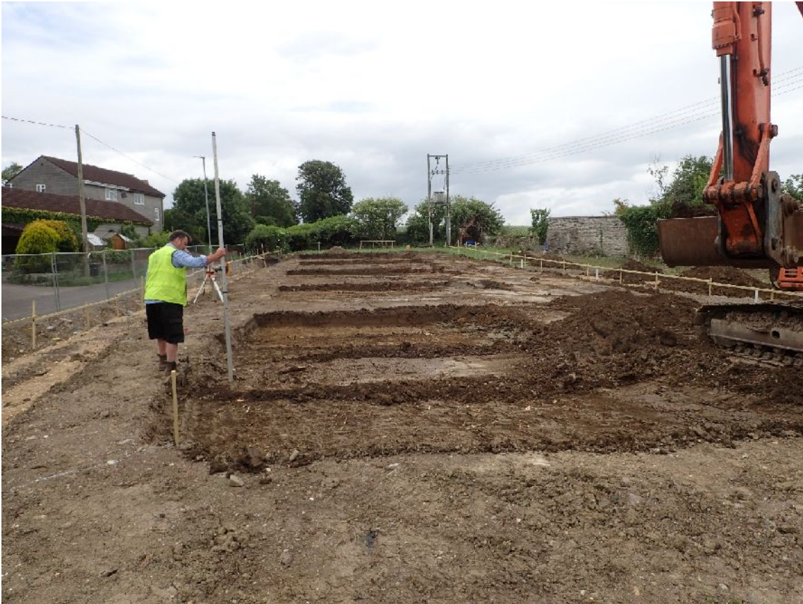
Plate 1. Working shot: excavation of terraces for house platforms (from SSW, no scale)
