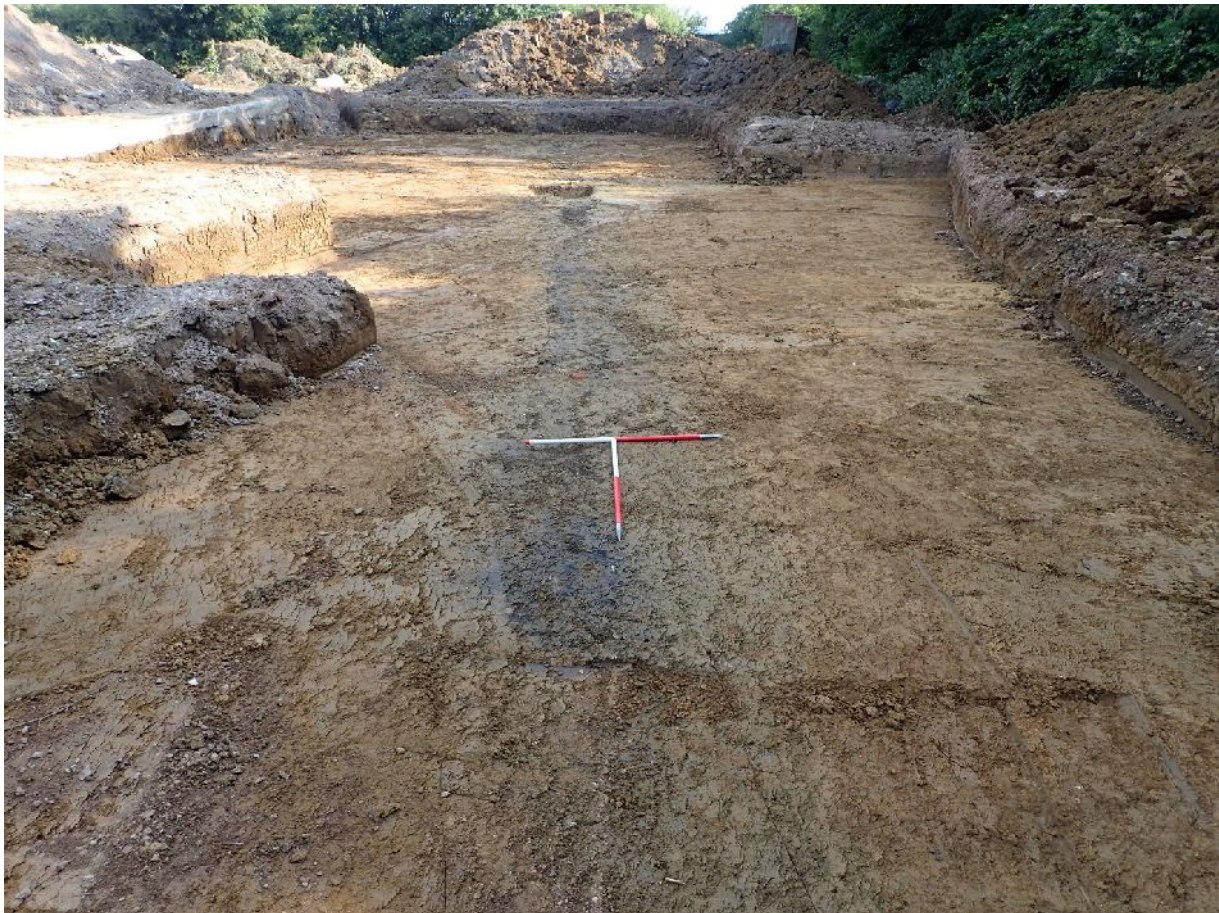
Plate 3. Line of ditch (F1) with excavated section in the background (from SSE, 2 x 1m scales)
