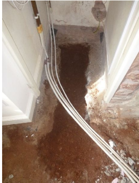
Plate 2. Boiler cupboard area (facing W)
