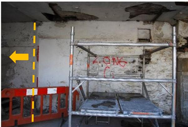
Plate 5. B1 Wall A ground - between 17 th century fireplace & east end showing curve in wall (from N)
