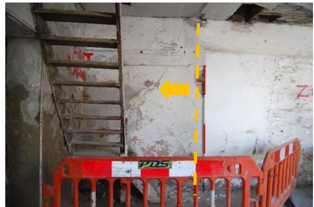
Plate 6. B1 Wall A ground - east end showing curve in wall (from N)
