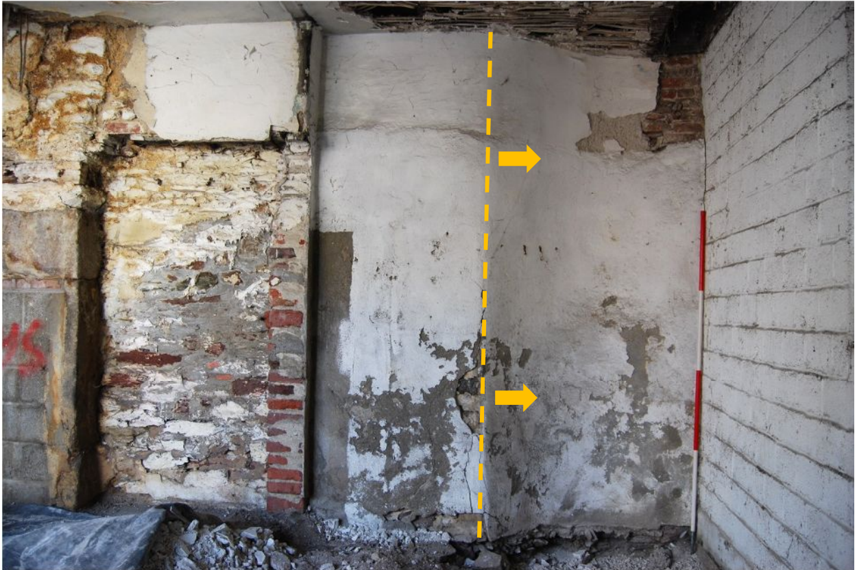
Plate 4. B1 Wall A ground - 17 th century stair turret at west end (from N)
