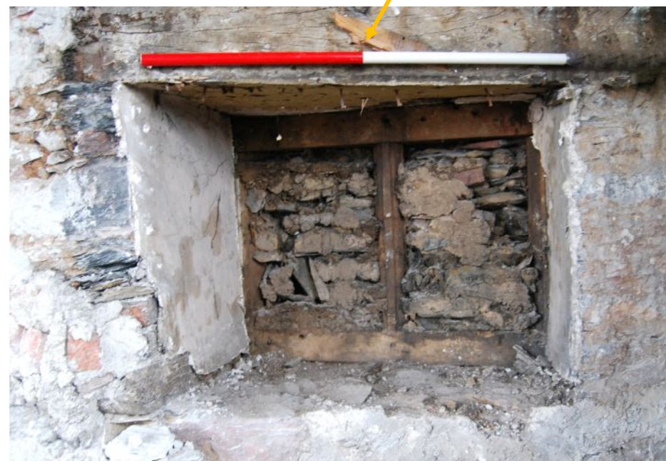
Plate 10. B1 Wall A first floor – late 17 th to early 18 th century window (from N)
