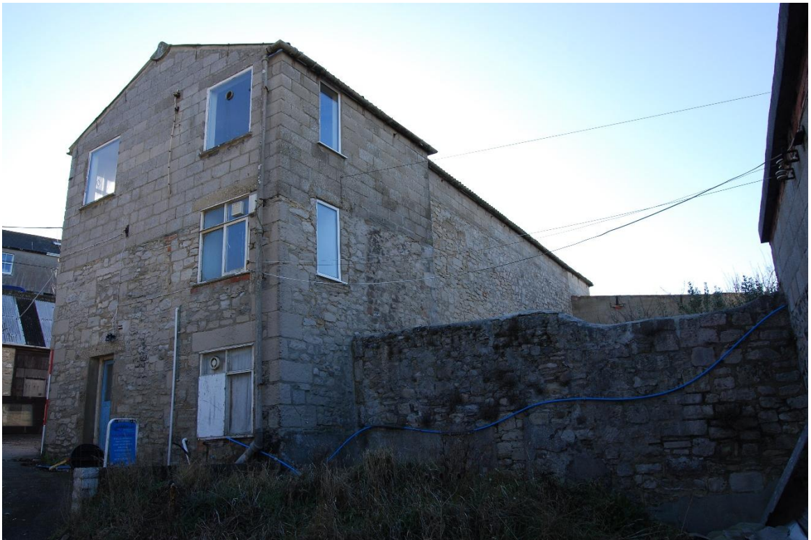
Figure 20. North end & west facing elevation of building A (2m scale, looking SE)
