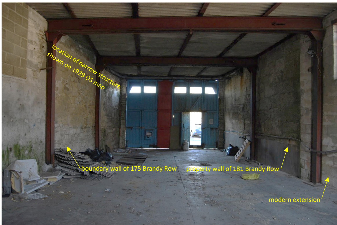
Figure 12. Building F with side walls formed by adjoining properties (2m scale, looking W)
