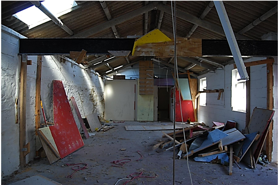
Figure 23. Upper storey of building A, accessed from north end of building (2m scale, looking N)
