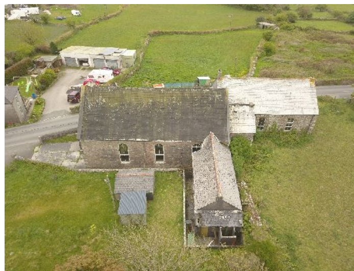
Plate 16. NE side showing extension with lean-to & retaining wall around walkway (from NE)
