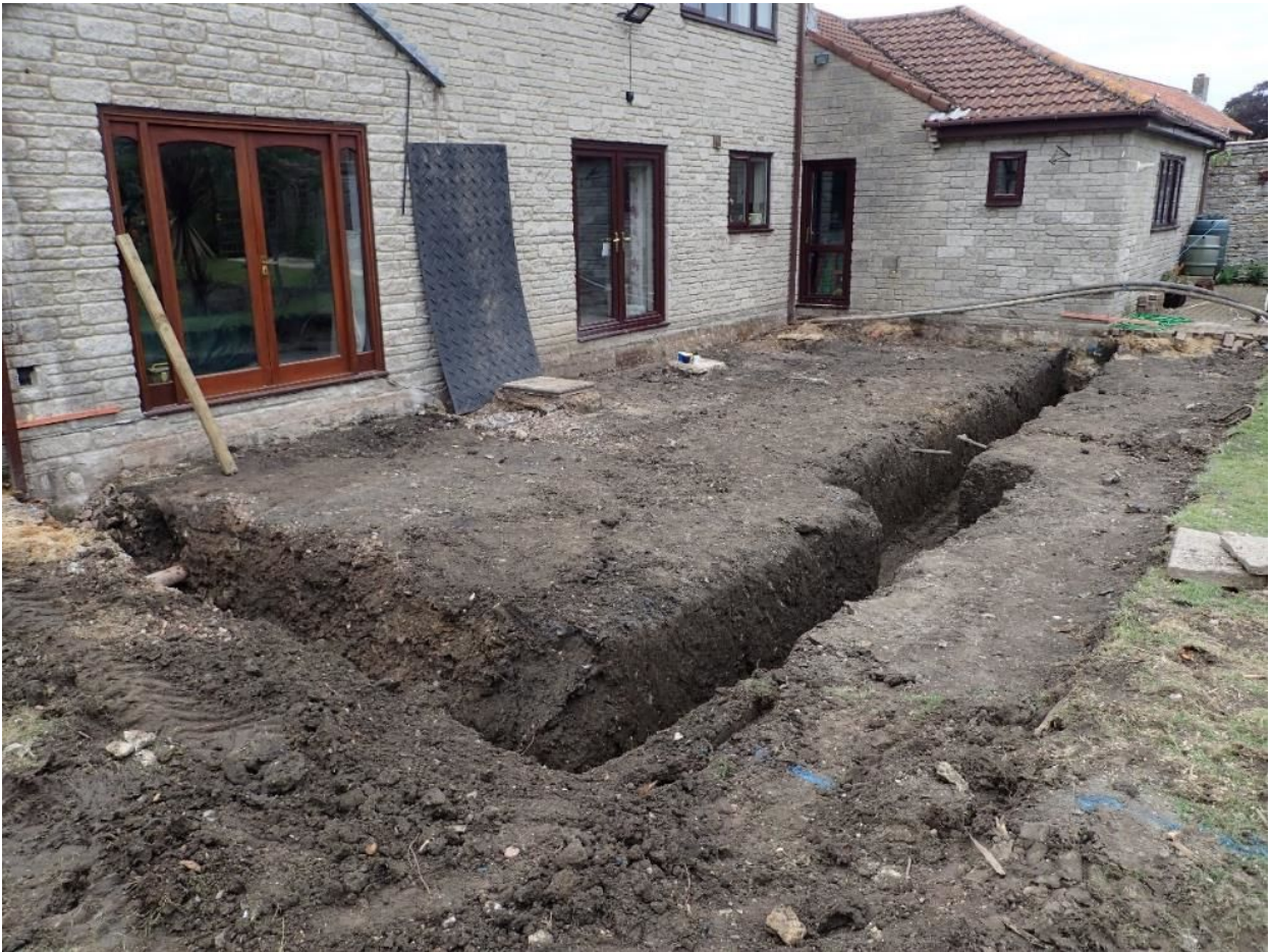
Plate 1. General view of the excavated foundation trenches from the south (no scale)
