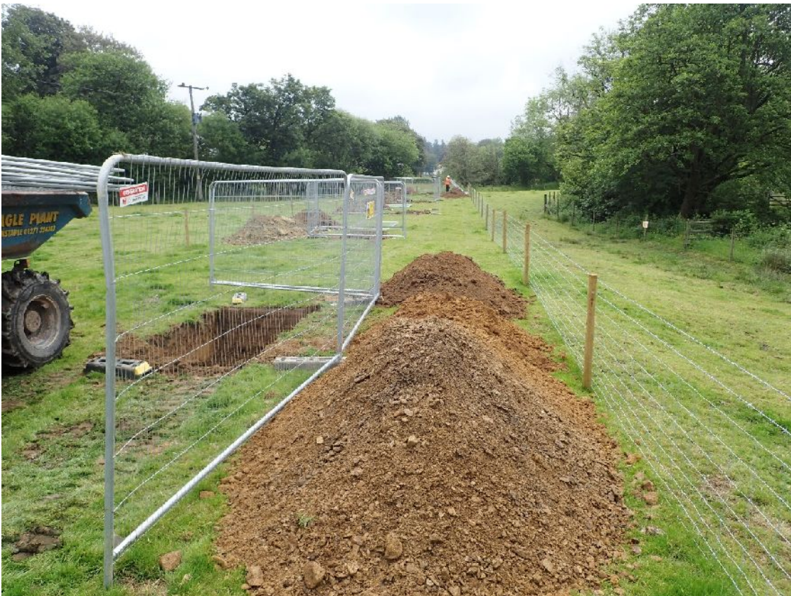
Plate 2. General view across the Site showing distribution of directional drill pits from the north-west
