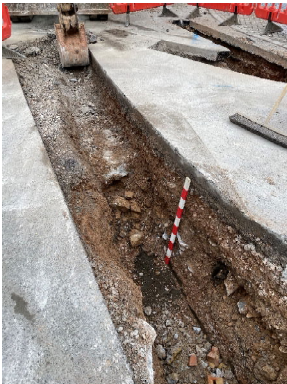
Figure 5. Service trench excavations showing buried soil in deepest part of trench (1m scale, looking W)
