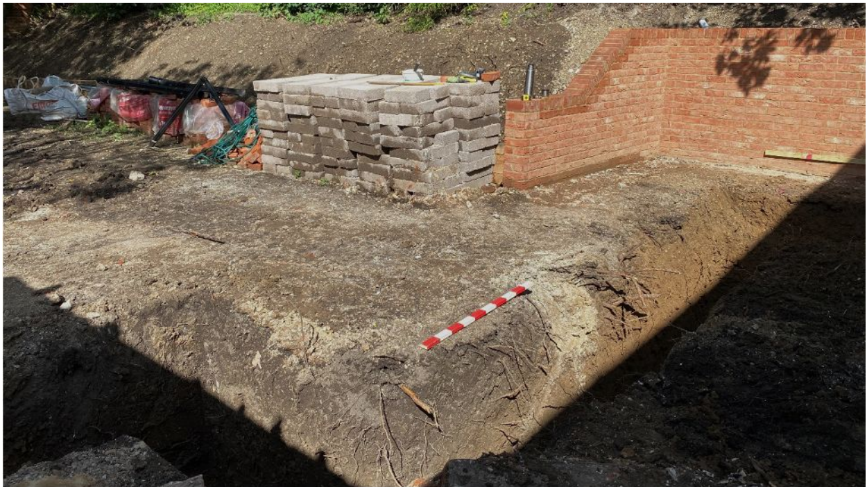
Figure 3. Foundation trenches for new extension at northern end showing bank and terracing (view from SW, 1x 1m scale)
