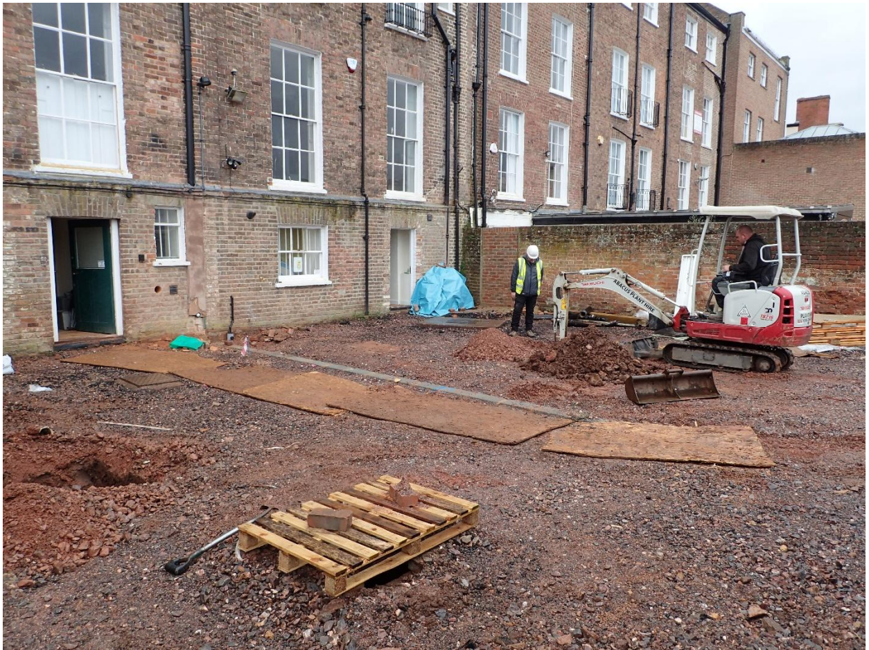
Figure 2. General view across site showing the excavated stanchion pits (no scale, from SE)
