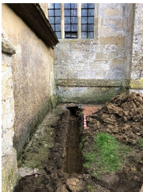
Figure 4. Service trench along W side of N porch (from N; 1m scale)
