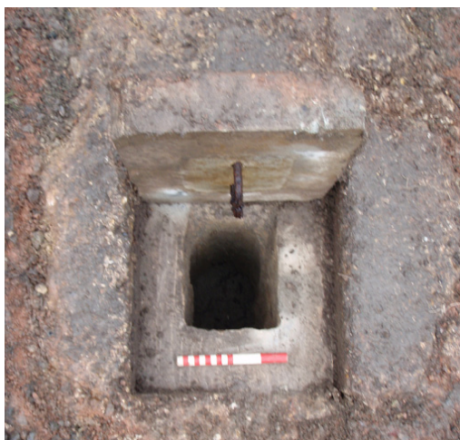
Plate 4: Concrete cover lifted showing socket into which a rigid steel girder could be inserted
