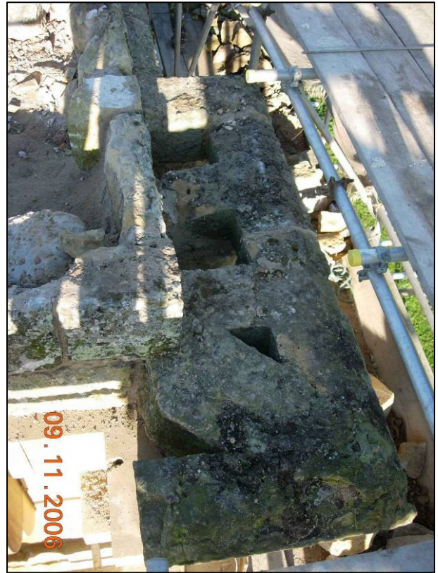
Plate 12: Detail of machicolations, prior to repair (photo courtesy of HPR).
