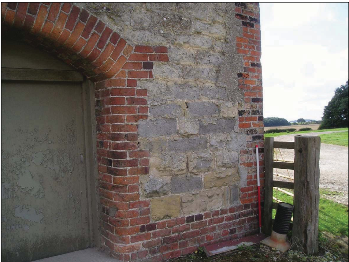
Plate 2: Brick quins and arch detail in north-west corner of cart shed, looking SW (photo 3/92).
