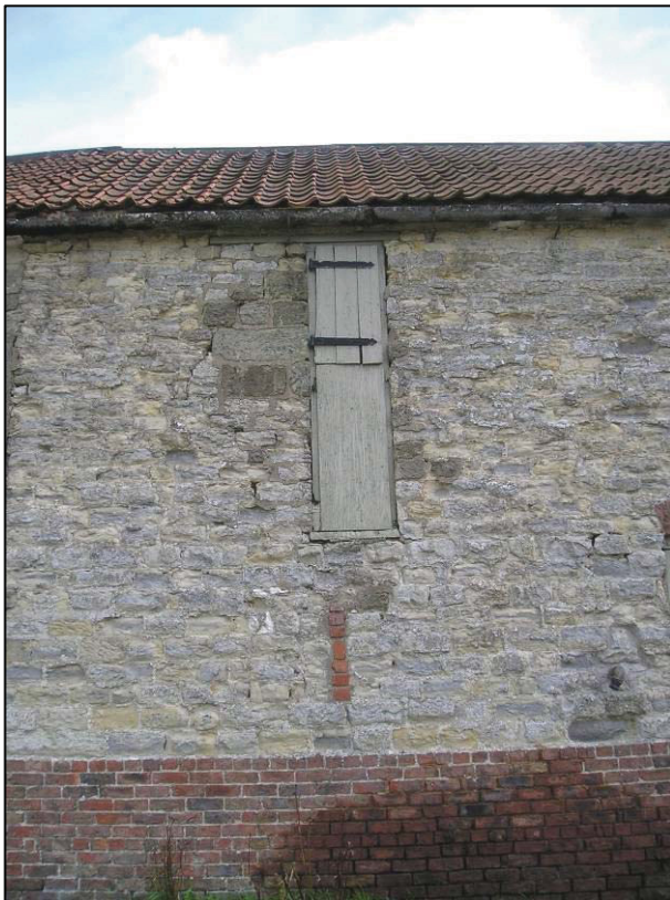
Plate 9: Possible belt drive opening, north end of west elevation of barn, looking E (photo 3/48).
