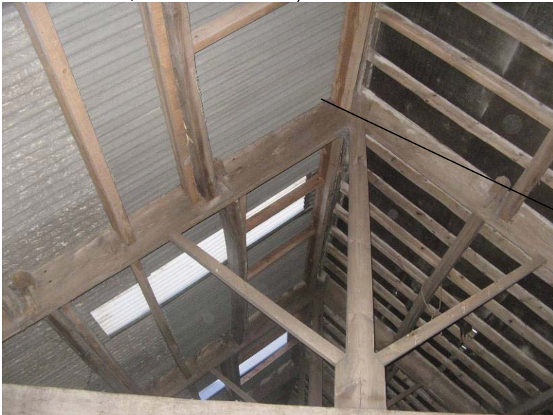
Plate 4 Location of bat roost within the first floor of Barn A (looking towards the third king post and principal rafter, from the stairwell)
