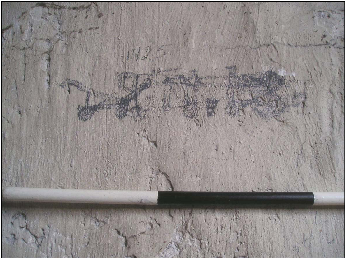
Plate 6: Sketch graffiti of threshing machine and elevator, dated 1925, on north wall, first floor of cart shed (photo 3/64).
