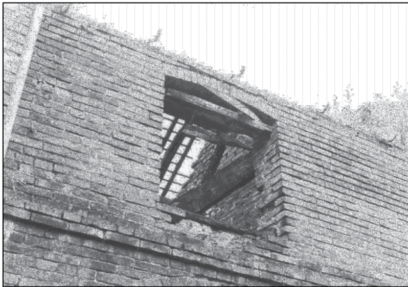
Plate 67: Building C, 1F truss over N 1F cell, viewed through 1F window in E elevation, looking W (photo 2/11).
