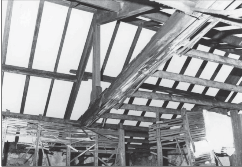
Plate 129: Building D, roof truss, S wall of S 1F room, looking W (photo 5/9).
