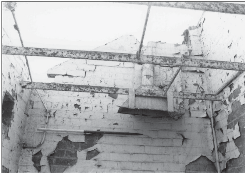
Plate 35: Building A, 1F SE corner room, detail of roof structure, looking S (photo 8/4).
