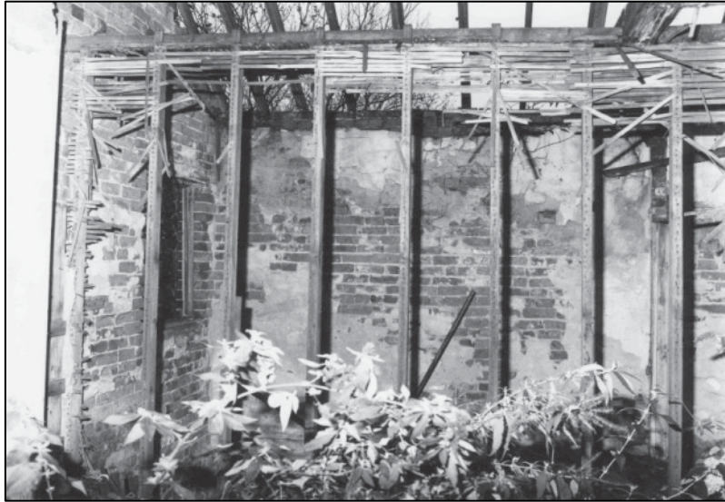
Plate 125: Building D, former partition, S wall of S 1F room, looking W (photo 5/7).
