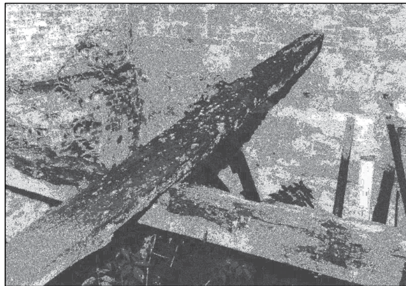
Plate 78: Building C, fallen timbers, N 1F room, looking SW (photo 4/10).
