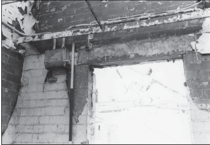
Plate 33: Building A, 1F SE corner room, detail of rail over door, looking N (photo 8/6).
