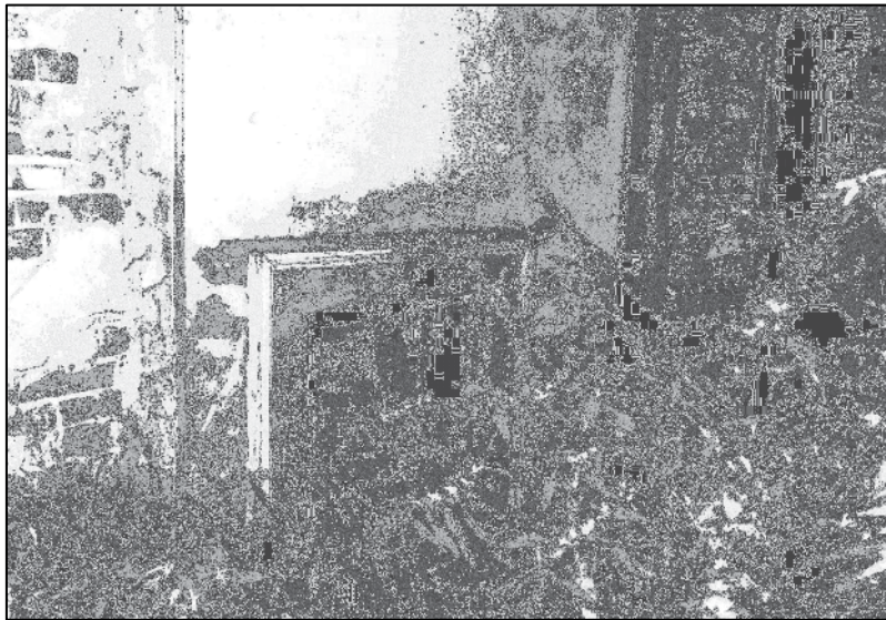
Plate 127: Building D, fireplace in S wall of S 1F room, looking S (photo 5/6).
