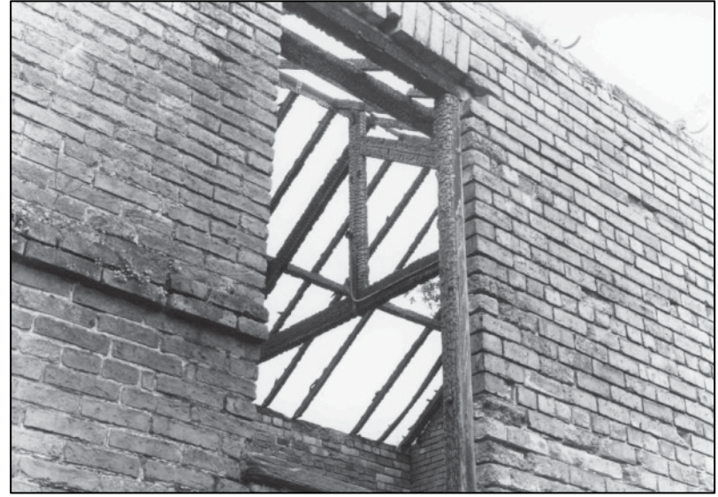
Plate 46: Building B, 1F truss viewed through 1F window in E elevation, looking S (photo 2/10).
