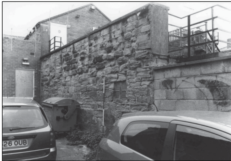
Plate 3: Stone wall to N end of yard wall to E of range, looking NE (photo 2/7).
