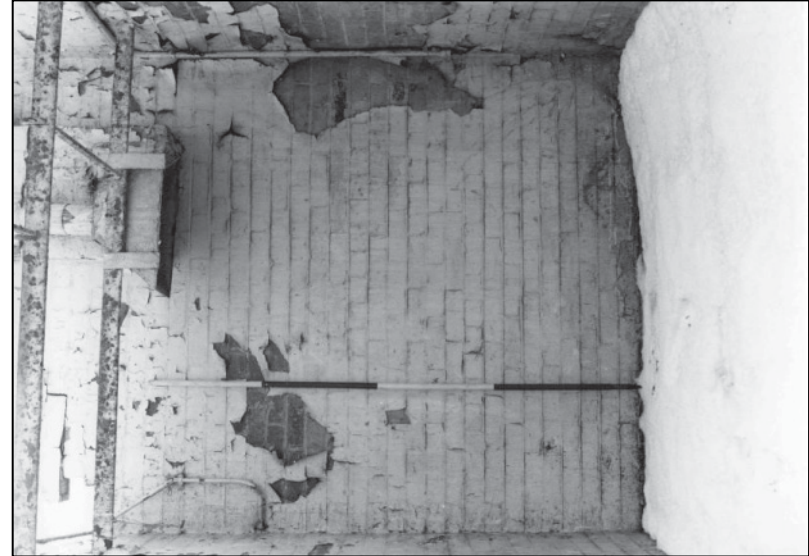
Plate 34: Building A, 1F SE corner room, looking S (photo 8/2) (top to left).
