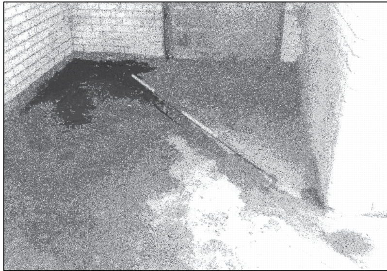
Plate 27: Building A, S part of GF, drain crossing floor, looking N (photo 9/10).
