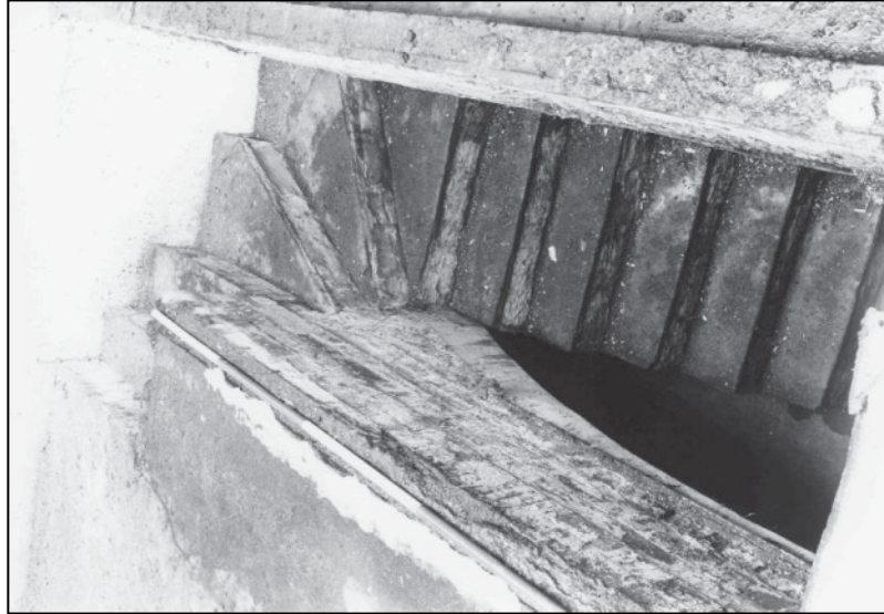
Plate 13: Building A, N part of GF, stairs to cellar, looking W (photo 10/5) (top to left).
