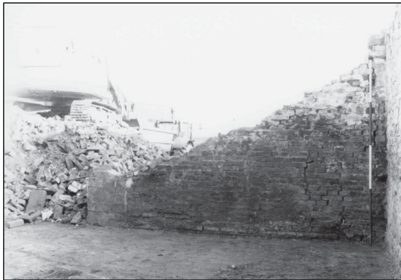
Plate 55: Building B, S wall of GF after partial demolition, looking SE (photo 10/13).
