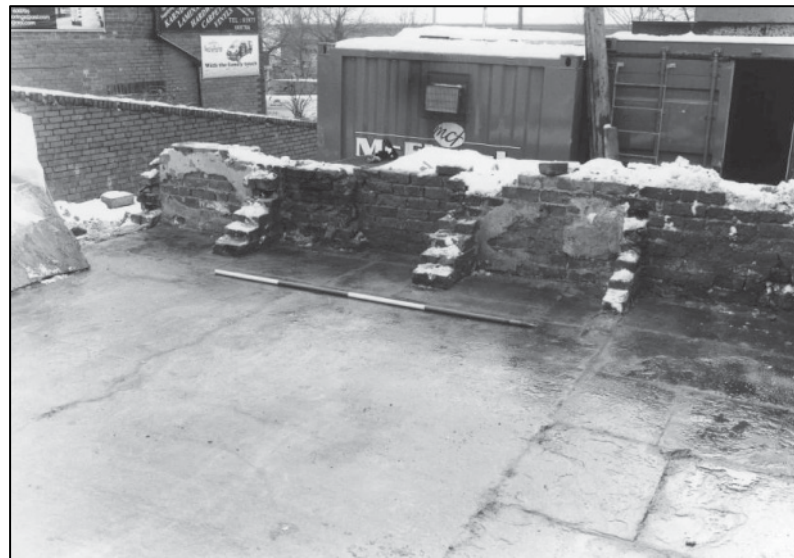
Plate 116: Building D, flagstone floor in S GF room, and stair after partial demolition, looking E (photo 6/17).
