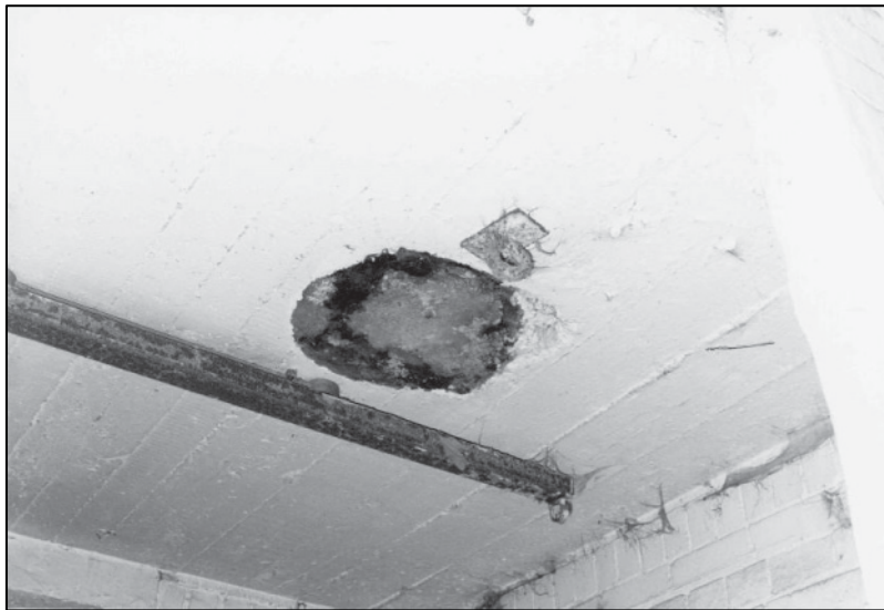
Plate 23: Building A, blocked hole and ring to ceiling, GF SE corner room, looking E (photo 9/2).
