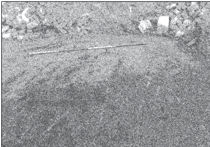
Plate 51: Building B, concrete floor of GF after partial demolition, looking E (photo 10/16).
