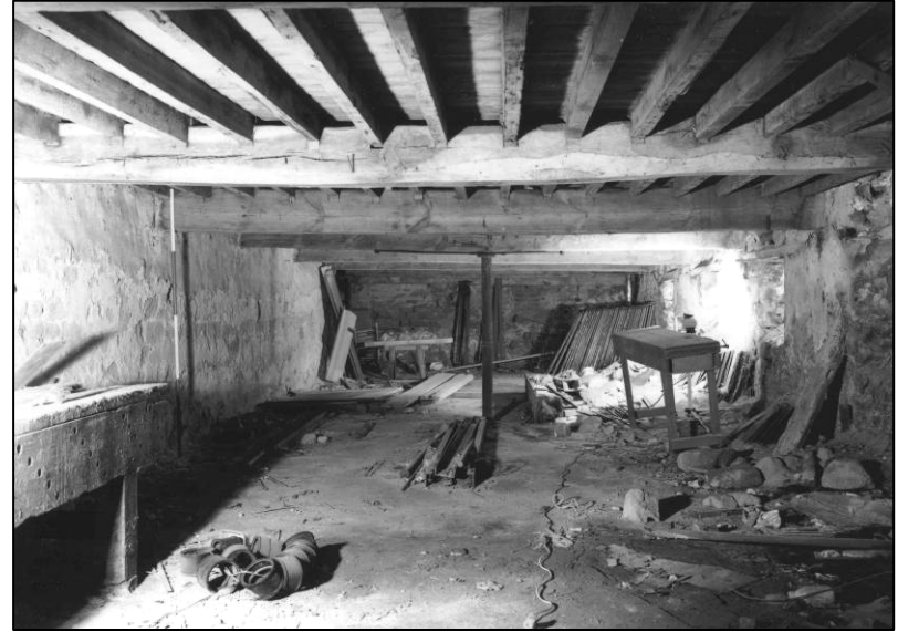
Plate 34: Ground floor area (central part), E of spine wall, looking NW (photo 3/13).
