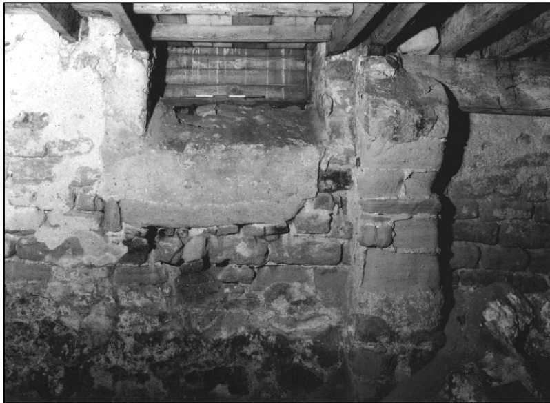
Plate 47: Doorway and arch in N wall, ground floor area W of spine wall, looking NW (photo 4/17).
