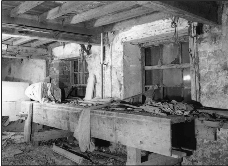
Plate 37: Joiner's bench and casement windows, W wall of ground floor area W of spine wall, looking S (photo 4/7).
