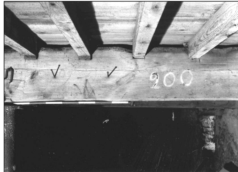
Plate 4: Typical painted numerals (200), ground floor area E of spine wall, looking NW (photo 4/5).
