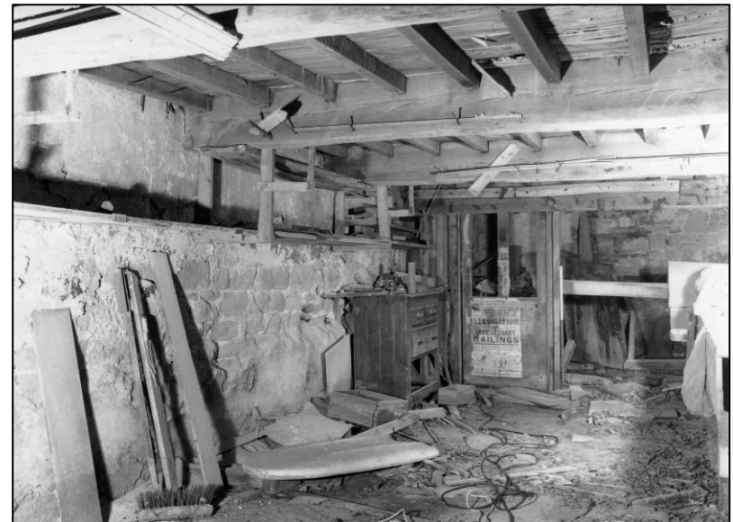
Plate 40: Ground floor area (S end), W of spine wall, looking SE (photo 4/10).
