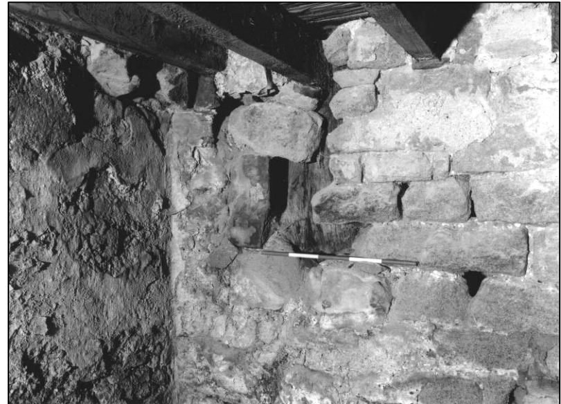
Plate 48: Timber buried in N wall of ground floor area W of spine wall, looking W (photo 4/18).
