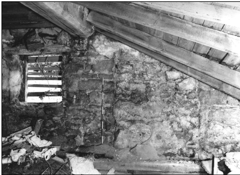
Plate 27: Blocked doorway, E wall of ground floor area E of spine wall, looking NE (photo 3/12).
