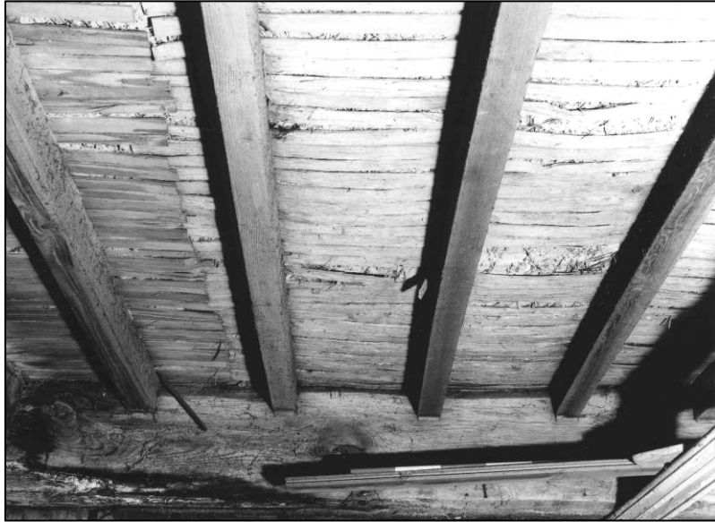
Plate 57: Underside of lath and screed floor over W side of building, looking W (photo 4/11).
