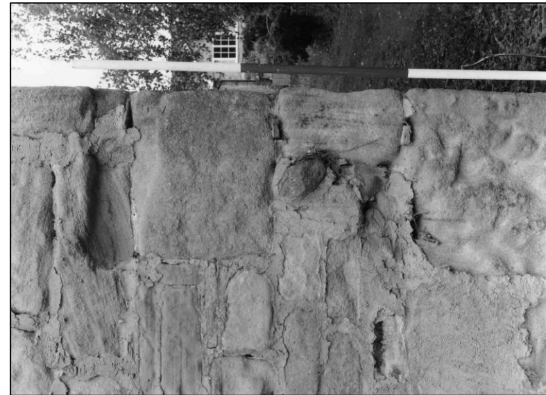
Plate 16: S gable, scar at E end left by removal of yard wall, looking NW (photo 2/12) (top to left).
