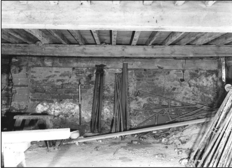
Plate 29: N wall of ground floor area E of spine wall, looking NW (photo 3/18).
