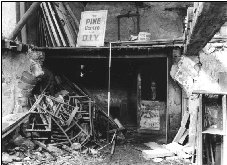
Plate 39: Wooden partition at S end of ground floor area W of spine wall, looking SW (photo 3/6).
