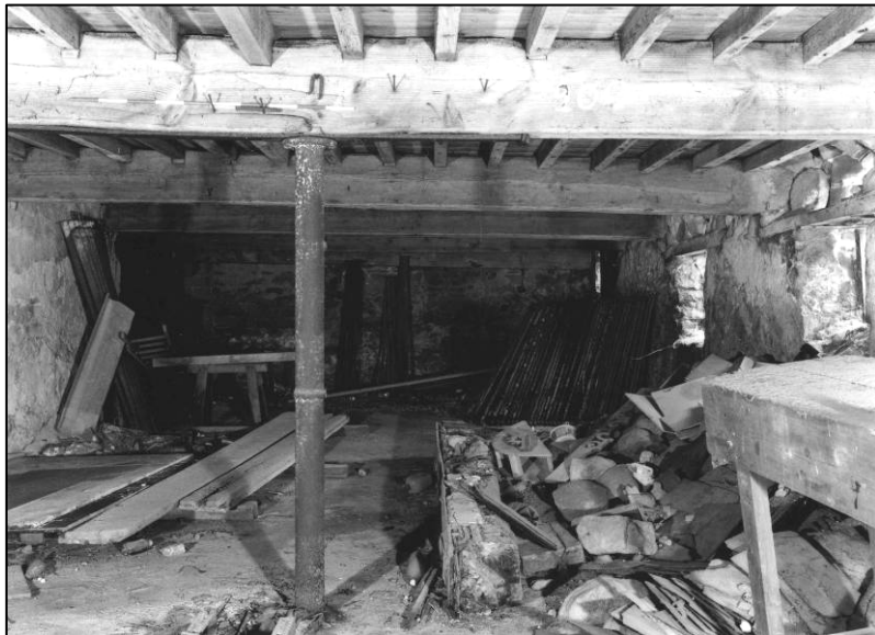
Plate 35: Ground floor area (N end), E of spine wall, looking NW (photo 3/17).
