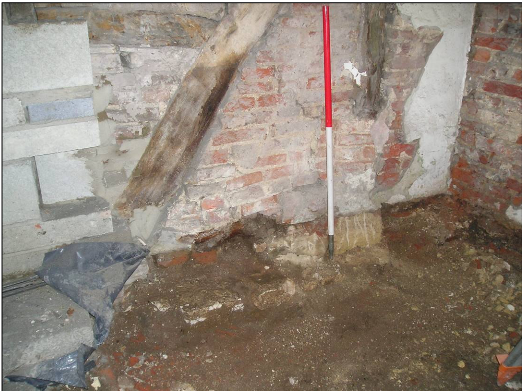
Plate 14: North wall of GF6 showing chalk and brick footings under framing, looking N (photo 38/22).
