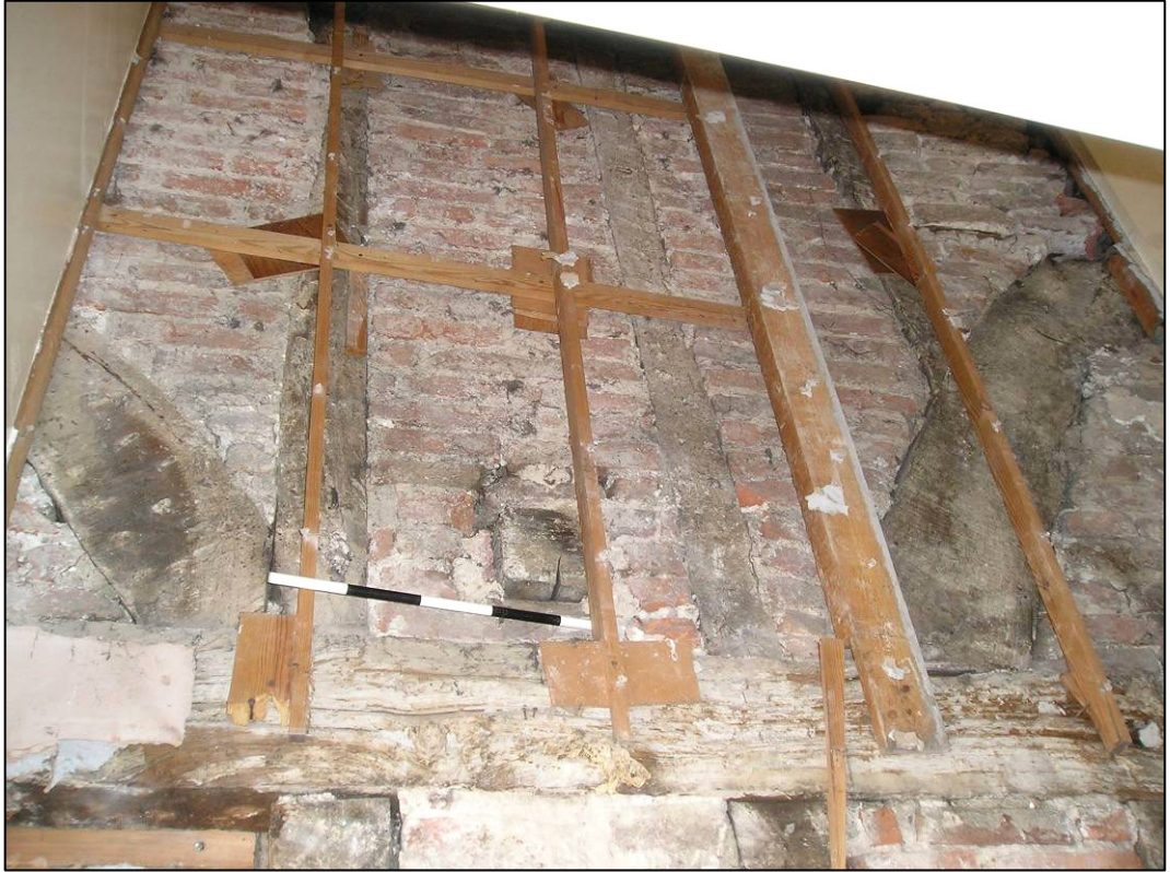
Plate 7: Framing to north wall of room 1F6 when first exposed, looking N (photo 31/20).
