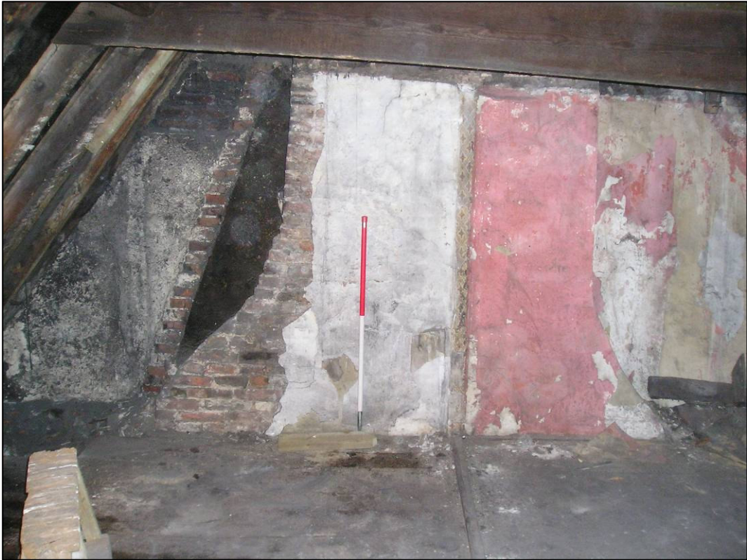
Plate 13: South wall of A3 after stripping out, showing firehood, looking SE (photo 38/6).
