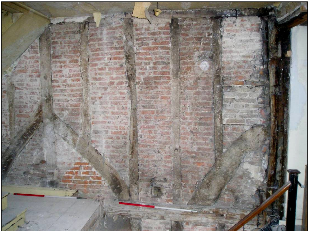
Plate 8: Framing to north wall of room 1F6 fully exposed, looking N (photo 32/1).
