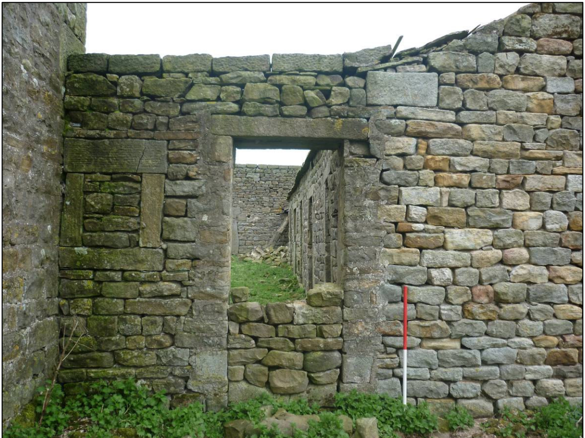
Plate 6: Doorway and blocked window in yard wall between east range and barn, looking N (photo 1/346).
