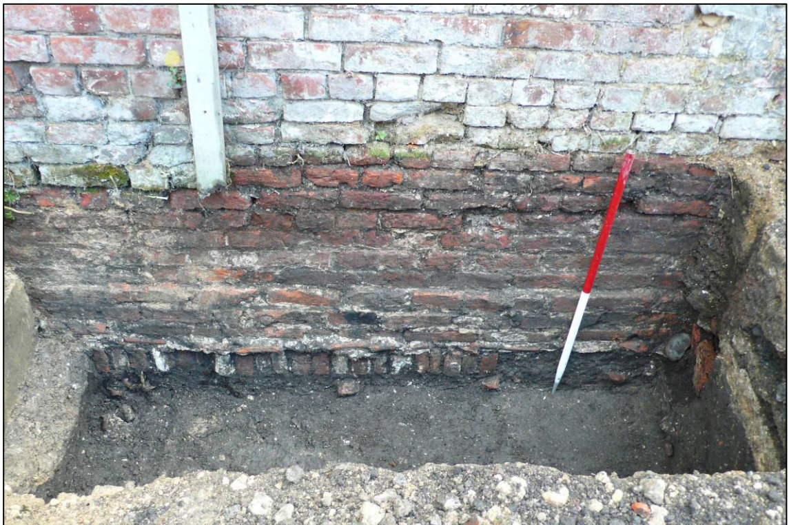
Plate 10: South side of drainage trench, showing wall (050) and foundation (051) of The Carriage House, looking S.
