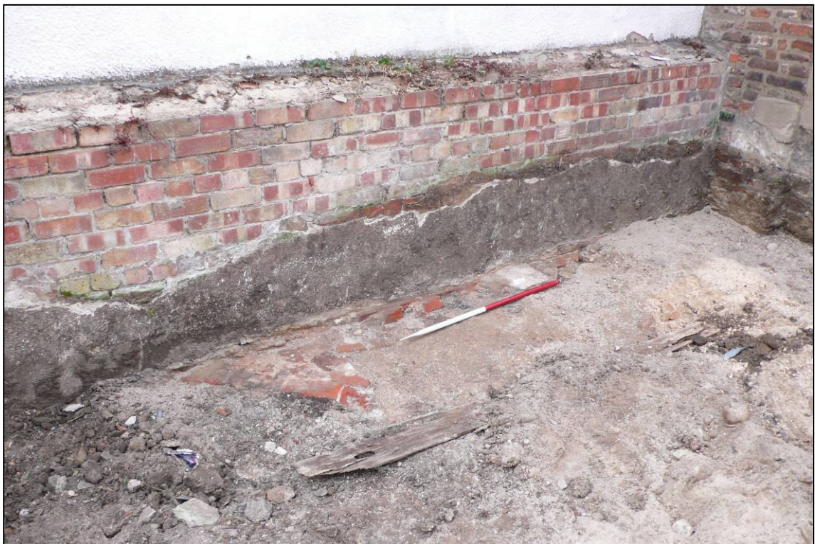
Plate 5: Remains of fireplace (014) and wooden plank (016), north side of site, looking N.
