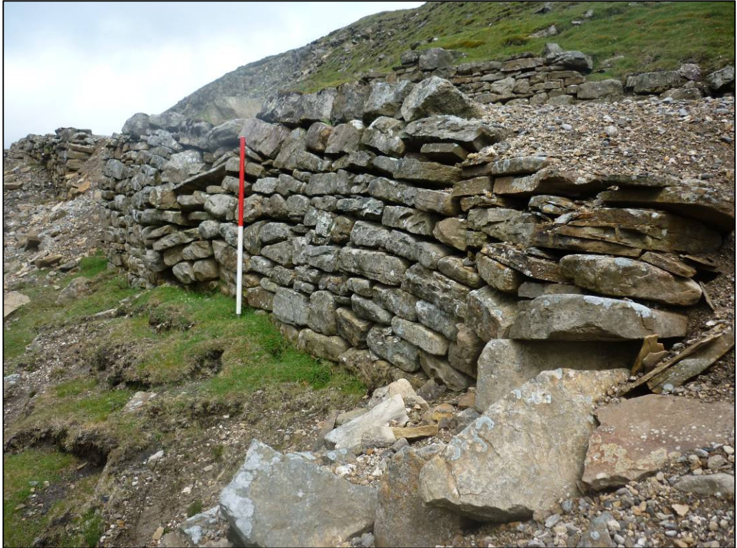
Plate 3: Central part of retaining wall between collapses, looking NW (photo 1/397).
