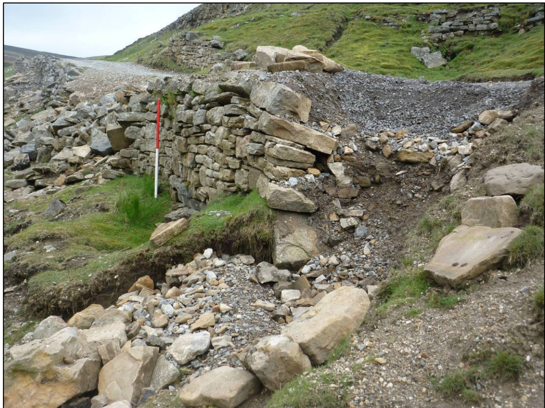
Plate 4: Collapse at east end of retaining wall, looking N (photo 1/399).
